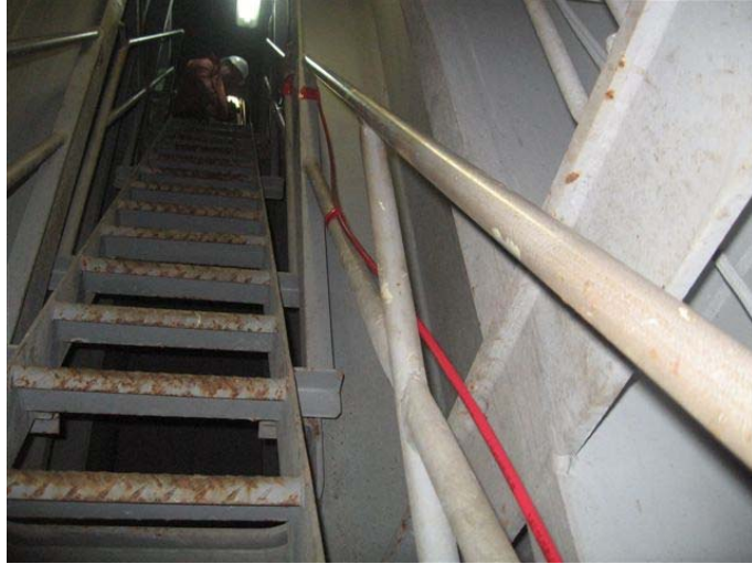
Picture 3.3.1 Tubing taped to hand rail in the stairway (viewing upwards)
