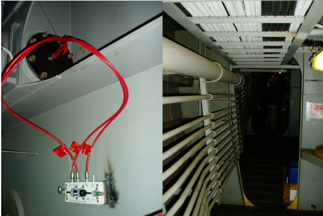
Picture 3.2.2 Feed through of tubing coming from cargo hatch in to the causeway with Sampling Panel A mounted on the wall. One tube is disconnected to show the white “parking” stud for the tubing. The right hand picture shows the under deck causeway
