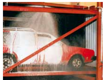
sprinkler system working
