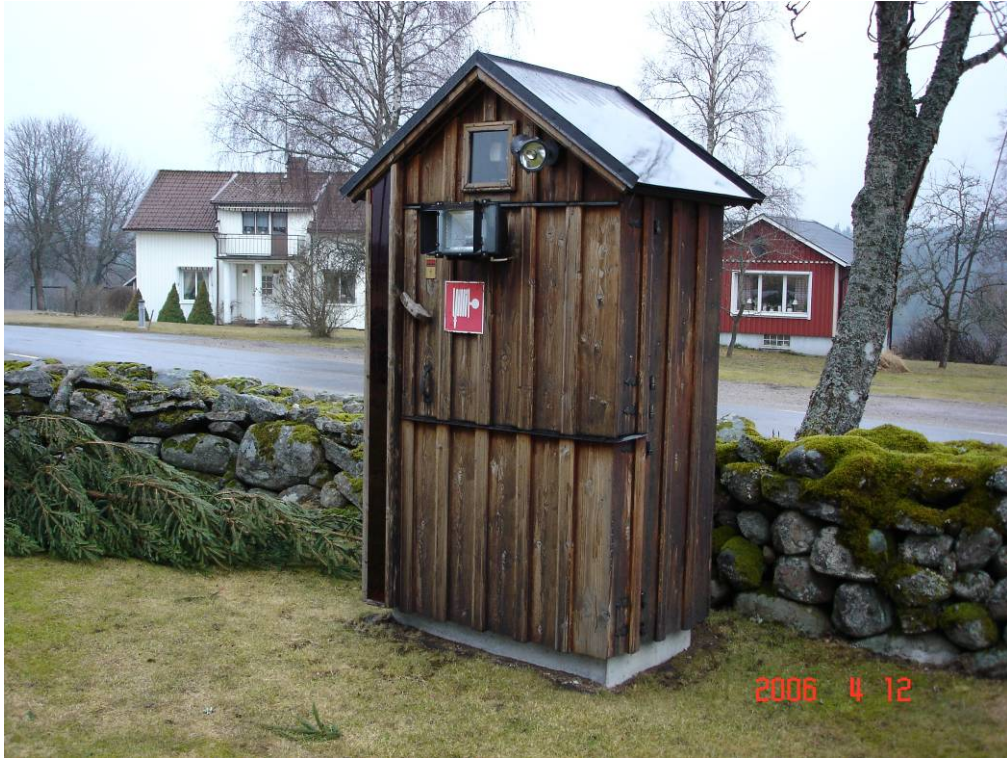
Insulated and heated cabinet containing a fire hose reel.
