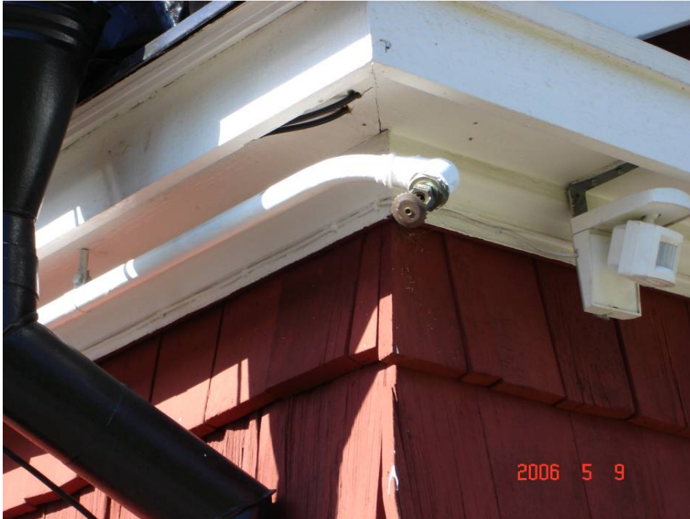
One of the (open) sprinklers used to protect the facade.
