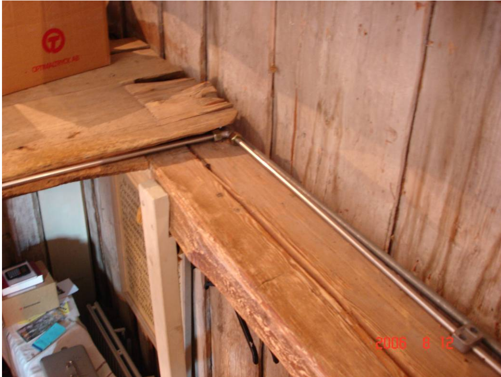
Visible but discreetly installed piping inside the church.
