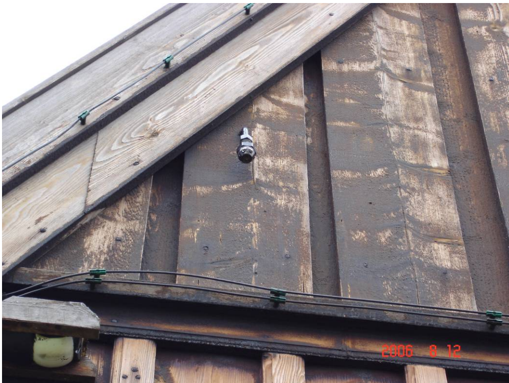
High-pressure water mist nozzle and linear heat detection wires on one of the facades.
