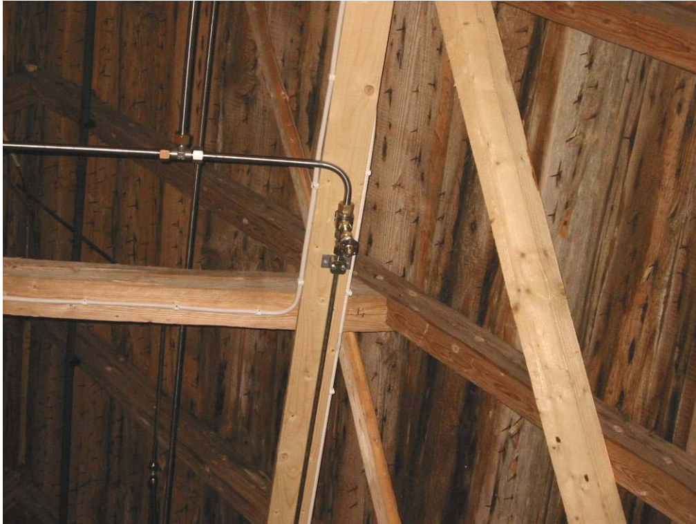
High-pressure water mist nozzle and pipe-work inside the attic of the church. Photo: Anders Lönnermark.
