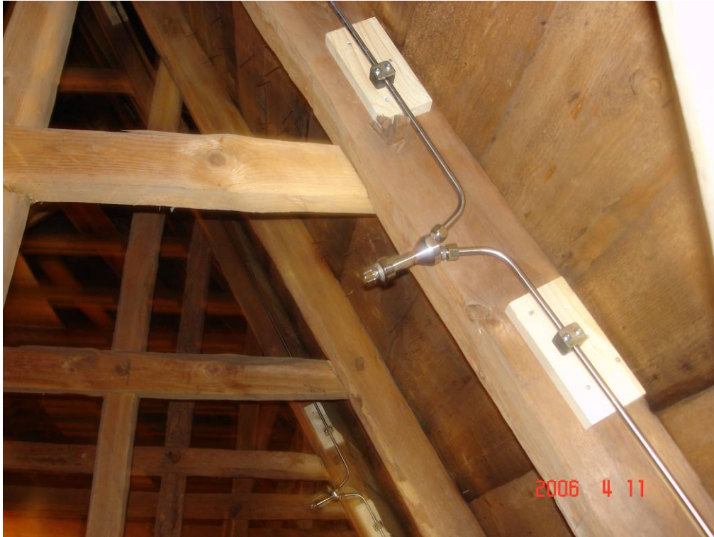
High-pressure water mist nozzles protecting the attic of the church. Note that Y-connection is used instead of a traditional T-connection. This connection limits the amount of standing water at the inlet of the nozzles and improves the possibilities to flush the piping with compressed air after an activation.
