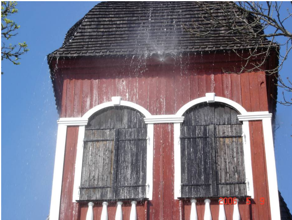
Functional test of the deluge system that protects the bell tower.
