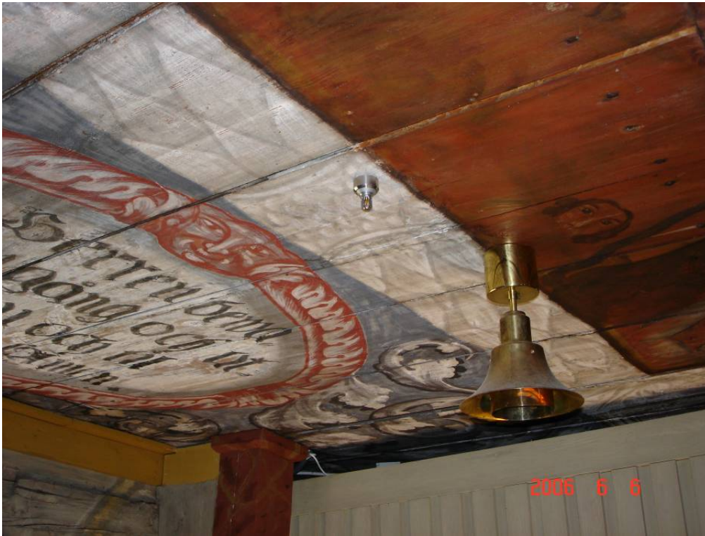
Figure 7 An automatic high-pressure water mist nozzle in Älgårds church. The position of a nozzle is often a compromise between fire protection, cultural historical and aesthetical demands.
