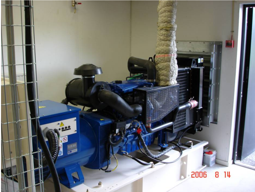
The diesel generator.
