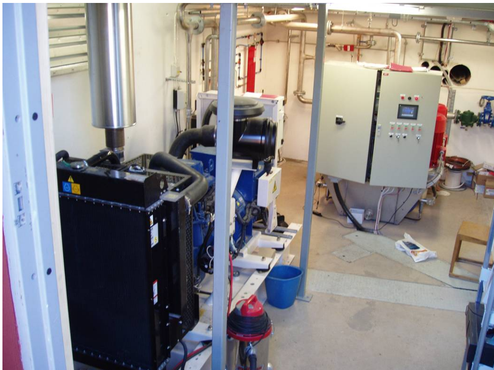
The high-pressure pump unit and the diesel generator (in front). Photo: Jan G Andersson.
