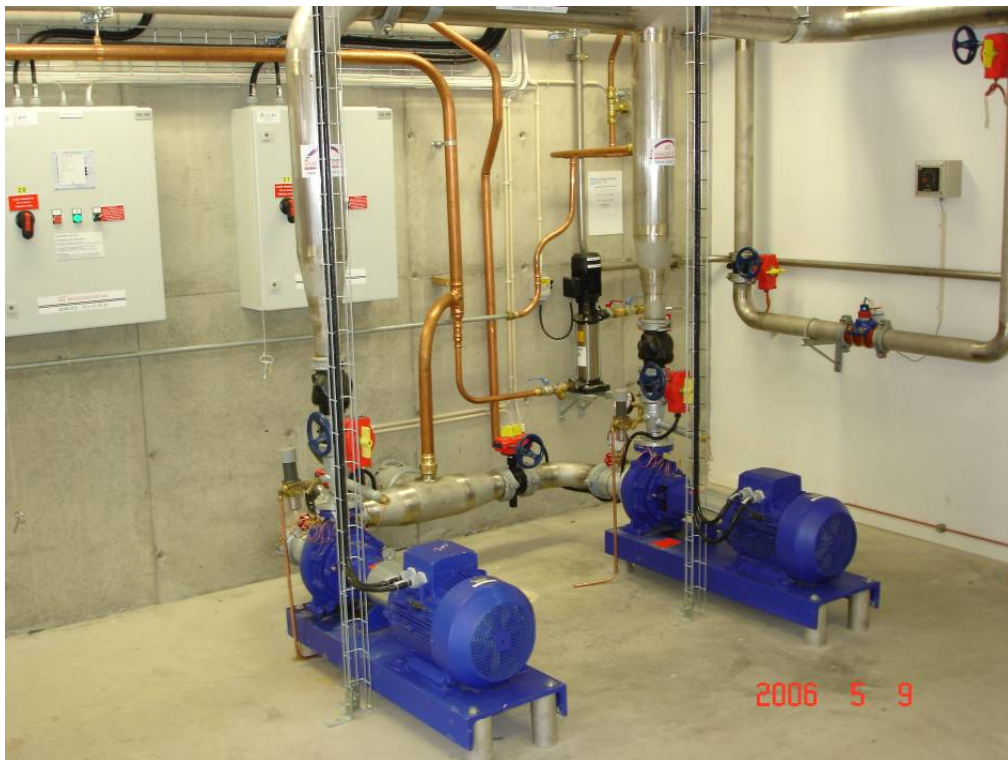
The electrical centrifugal pumps used for the low-pressure (sprinkler) system.
