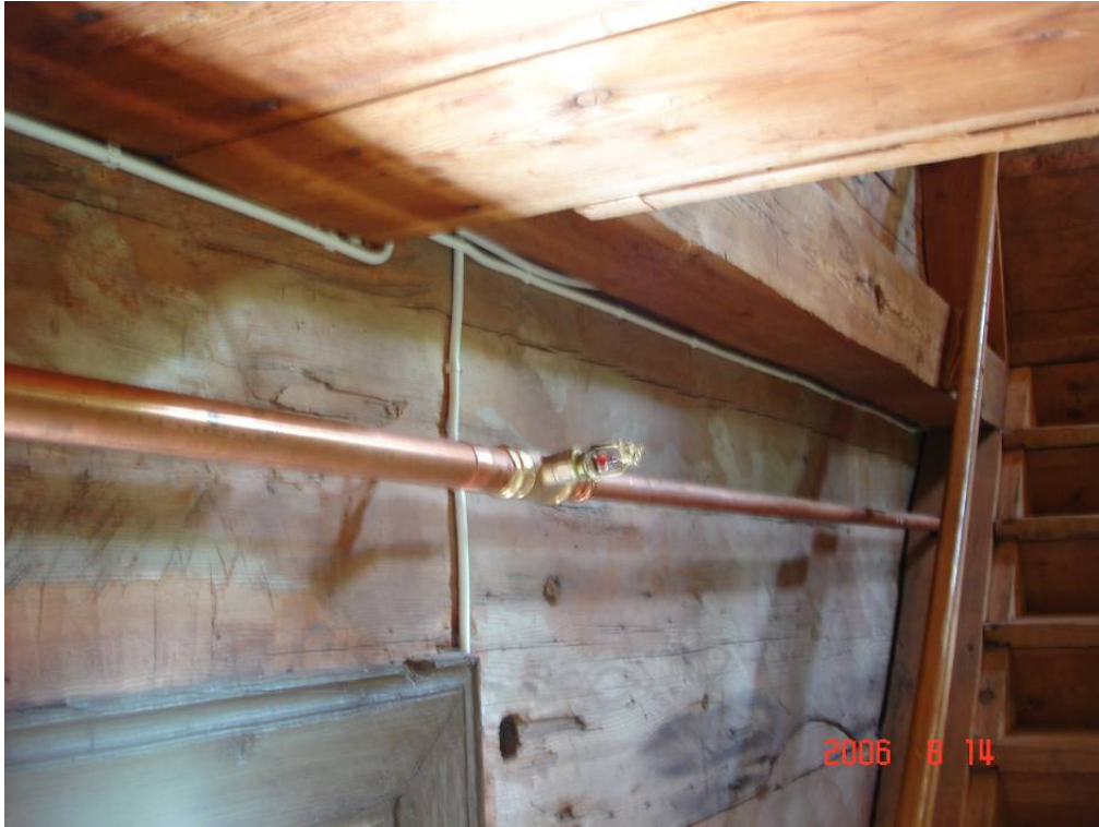
Sidewall sprinkler inside the church installed using copper piping.
