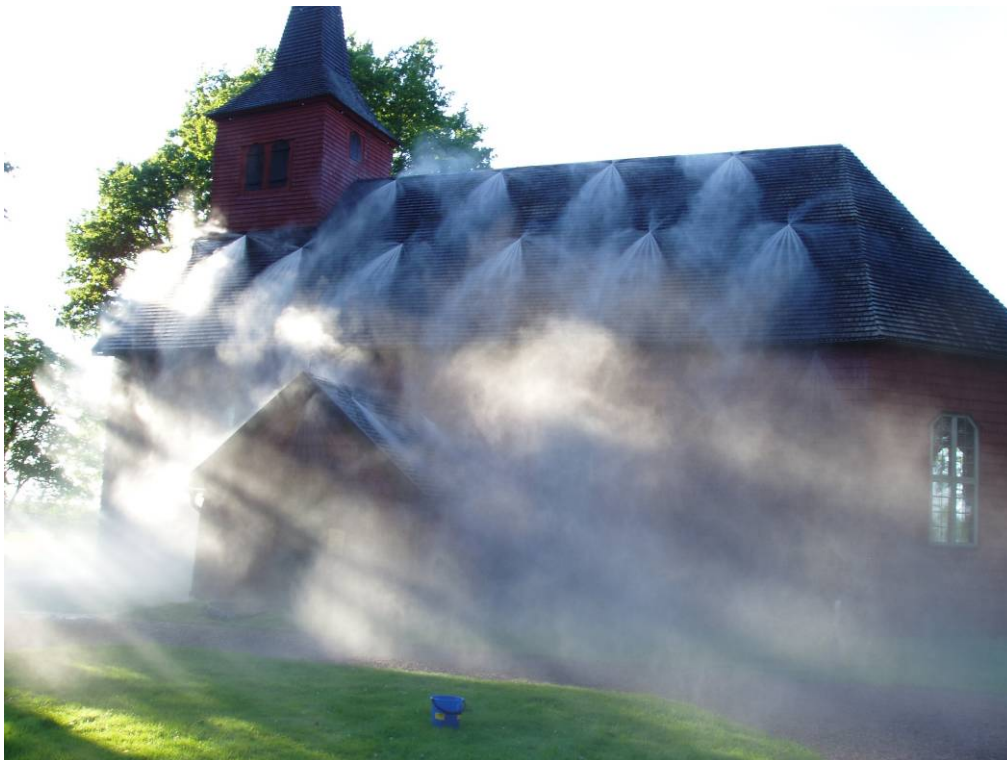
The picture shows a functional test of the system, where several sections that protects the facades and the roof was simultaneously activated. Photo: Jan G Andersson.
