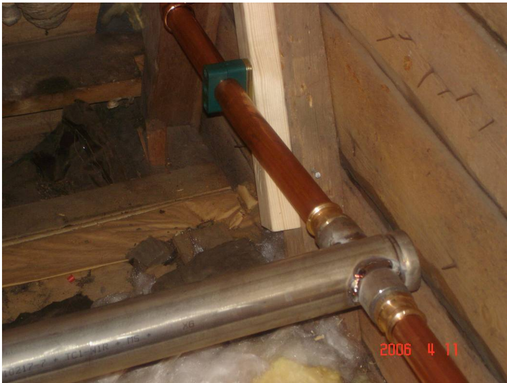
Pipe-work, inside the attic of the church, for the sprinklers protecting the facades. A stainless steel main pipe connects to the copper piping on the outside of the building.
