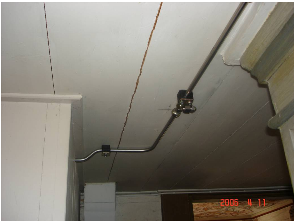
Visible, but discretely installed high-pressure piping.
