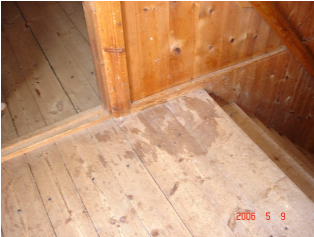
Figure 6 A spot on the floor at the Habo church caused by the leakage of the antifreeze solution used for (parts of) the sprinkler system.
