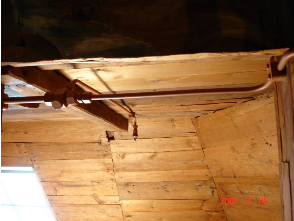
Some of the piping could not be concealed, but are discretely installed.
