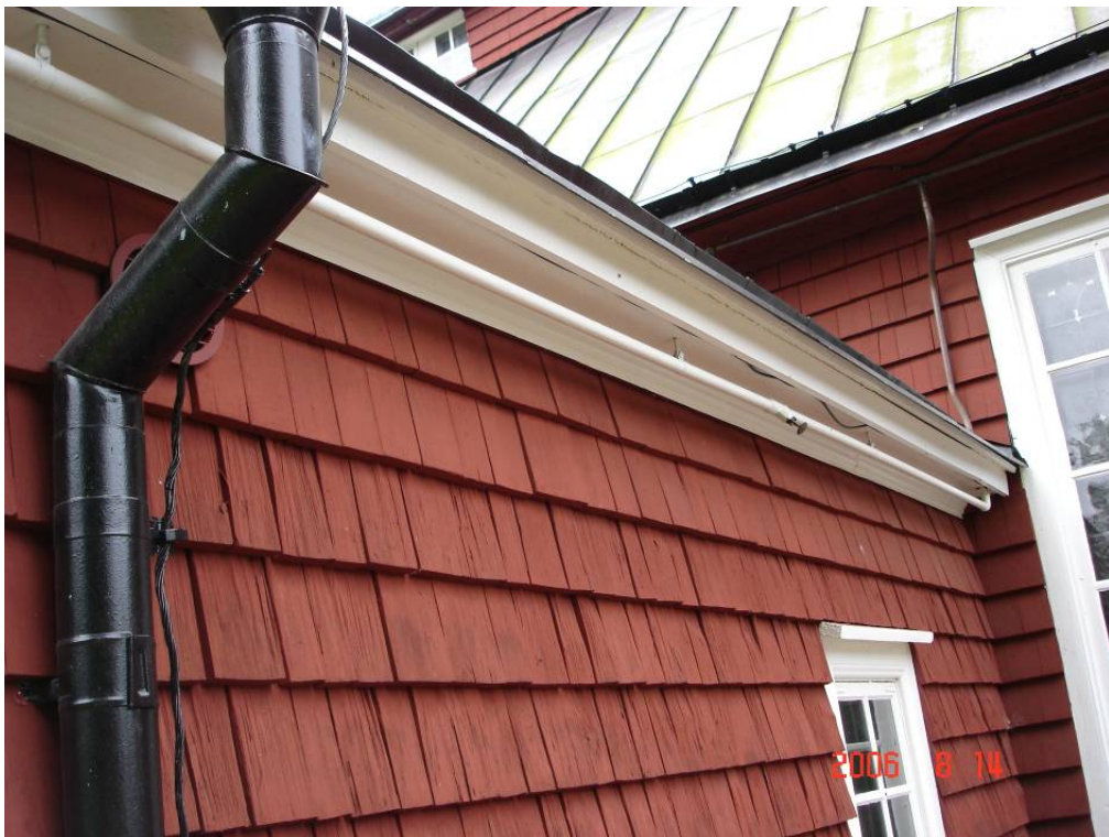
Sprinkler (open) used to protect the facade, with the pneumatic linear heat detection lines.
