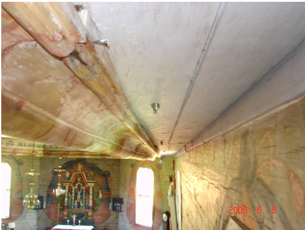
One row of automatic nozzles positioned close to a wall. These nozzles have a smaller K -factor as compared ( K=0,8 ) as compared to the other nozzles used for the interior, in order to limit the amount that hits the walls paintings.
