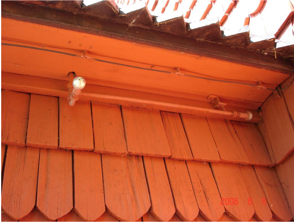
Two of the nozzles installed to protect the facade; the nozzle to the right is directed towards the corner in order to achieve additional protection against fire spread up the corner walls. The piping has been painted red to make the pipe as discreet as possible. Note the linear heat detector wire.
