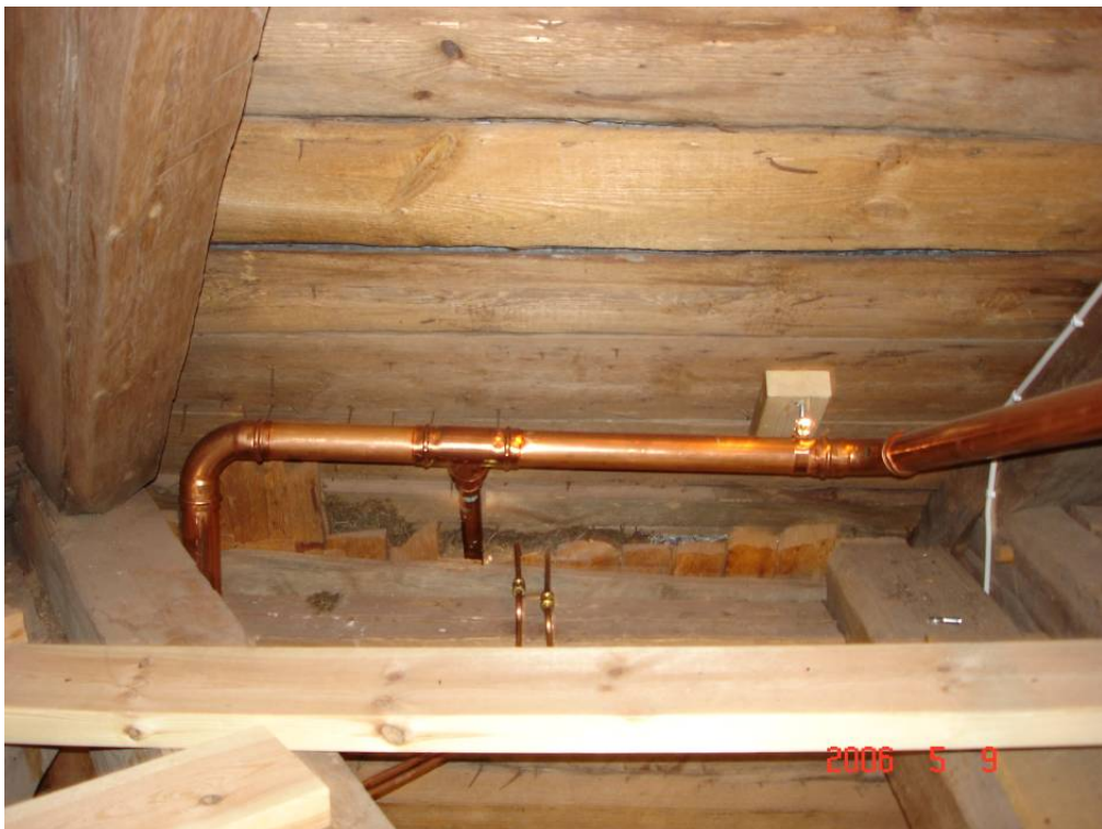
Photo from inside the attic. The copper piping connects to the pipe-work for the sprinklers protecting the facades. The smaller copper piping connects to the pneumatic linear heat detection system for the facades.
