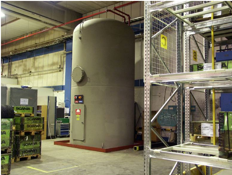
Figure 14 A 20 m 3 pressure tank used in an industrial application. The Nitrogen gas cylinders and the wet alarm valve are positioned at the bottom part, underneath the tank, with access through a steel door. Photo: Robert Linde.
