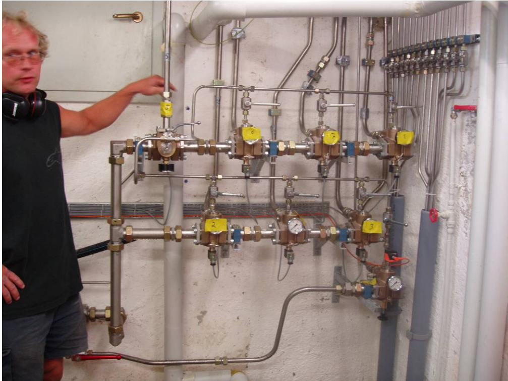
The section valves and the valves (at the right hand side wall) that are opened when flushing the system pipe-work with compressed air. All equipment is installed in the sacristy. Photo: Jan G Andersson.
