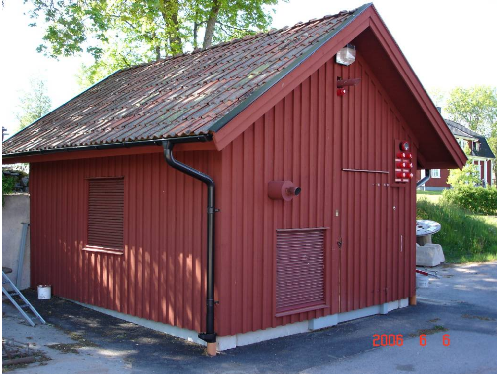
The newly built building close to the church that contains the pump unit, diesel generator and the fresh water tank. The building is insulated and heated.
