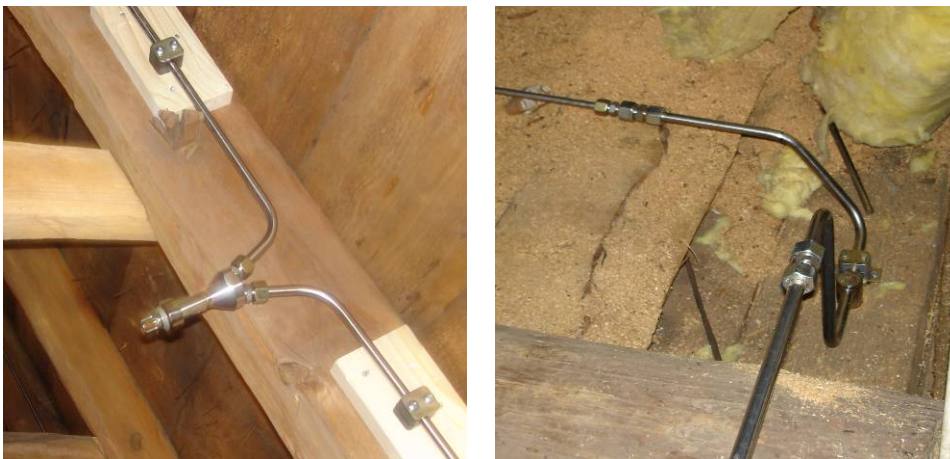
Figure 5 Y-connections are used to limit the amount of standing water at the inlet of the nozzles. To the left is shown an automatic nozzle inside the attic of Frödinge church. To the right, an automatic nozzle protecting the interior of Fröskog church, is shown.
