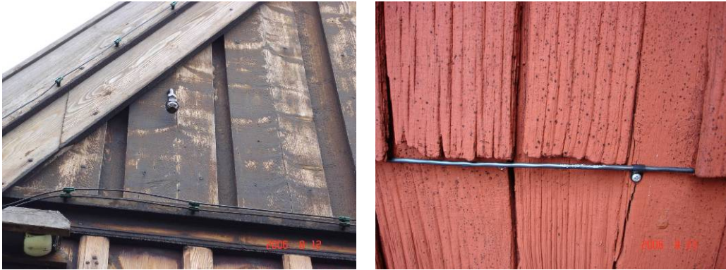
Figure 11 Linear heat detection wires at the facades of Hedareds stave church (left hand photo) and Fröskog church (right hand photo). Note the high-pressure water mist nozzle shown in the left hand side photo.
