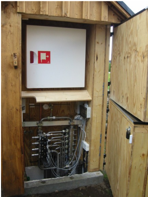
The inside of the cabinet containing the section valves and a fire hose reel. Photo: Anders Lönnermark.
