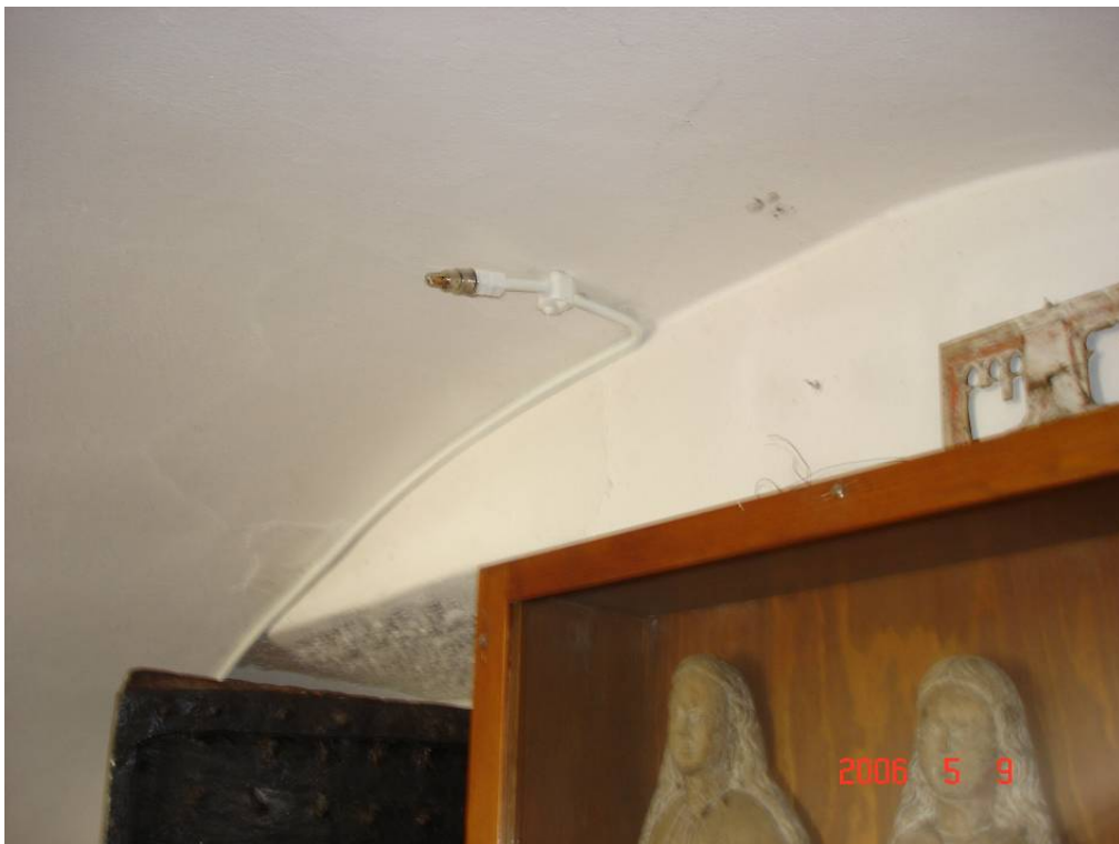
The small diameter piping typically used with high-pressure systems offers the possibility of discreet installations.
