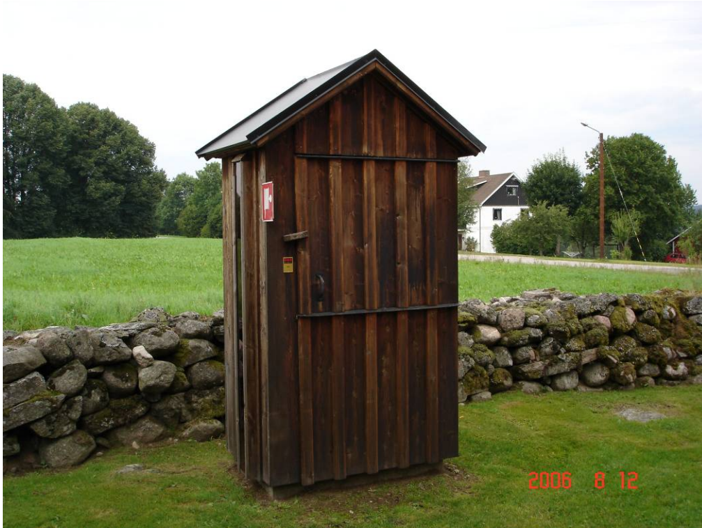
The insulated and heated cabinet containing the section valves of the system and a fire hose reel.
