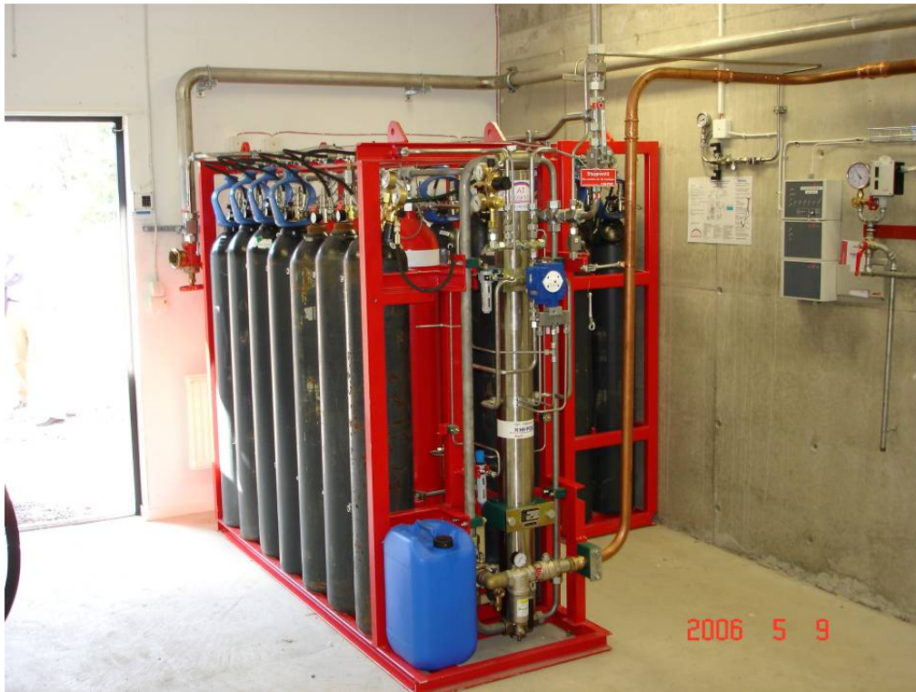
The gas driven pump (GPU) used for the high-pressure water mist system.
