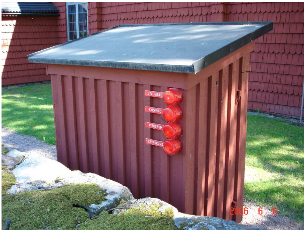
One of the cabinets that contains a fire hose reel. Indicator lamps on the cabinet show which part of the church was the source of the fire alarm.
