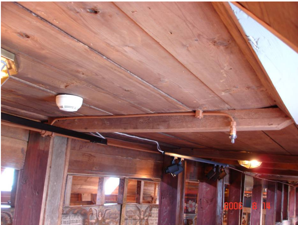
Figure 8 Sometimes, the sprinkler piping can not be concealed, but with the smaller diameter piping associated with high-pressure water mist systems, the installation can be made very discreet as in Habo church.
