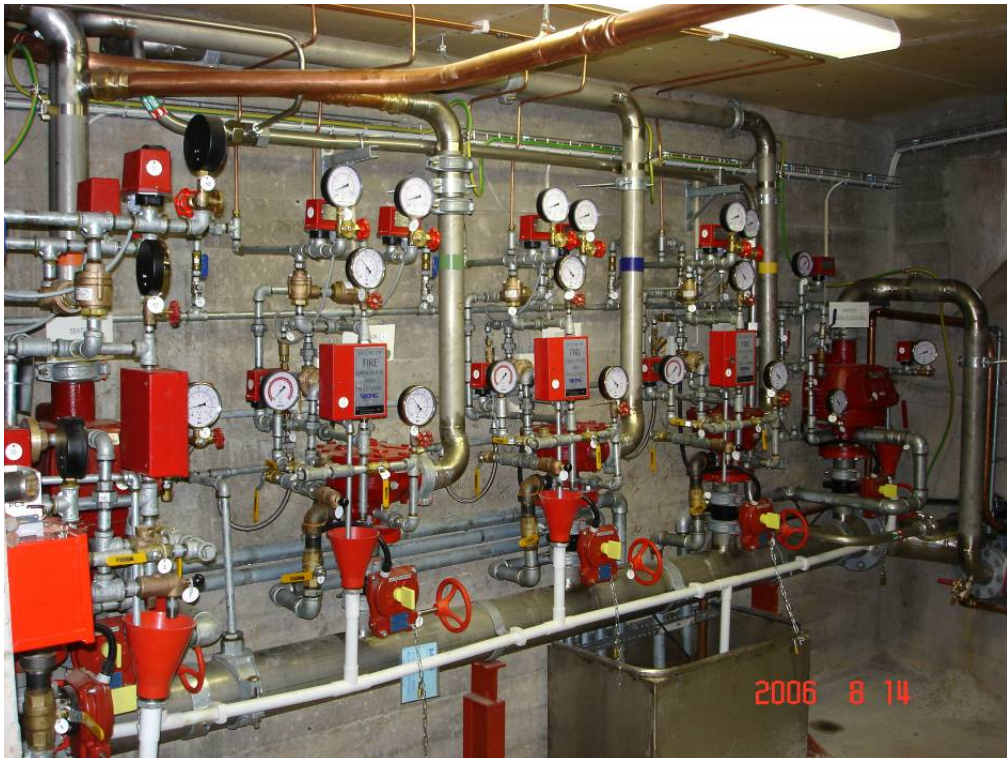
The deluge and dry-pipe valves used with the low-pressure (sprinkler) system. This equipment is positioned inside the church.
