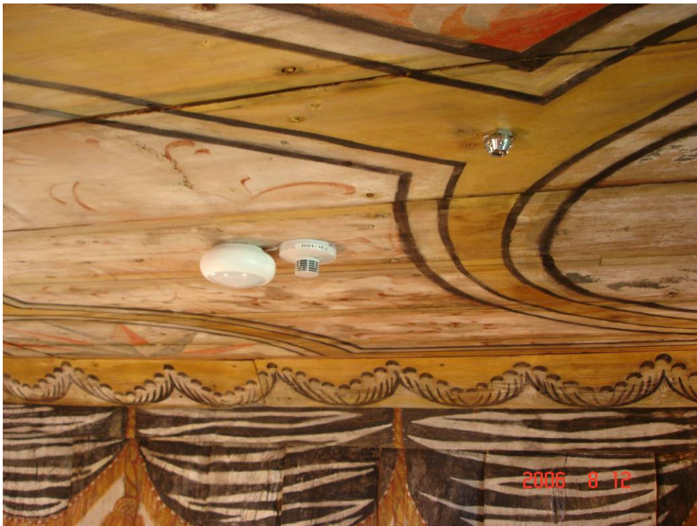
One of the high-pressure water mist nozzles and a fire detector at the ceiling.
