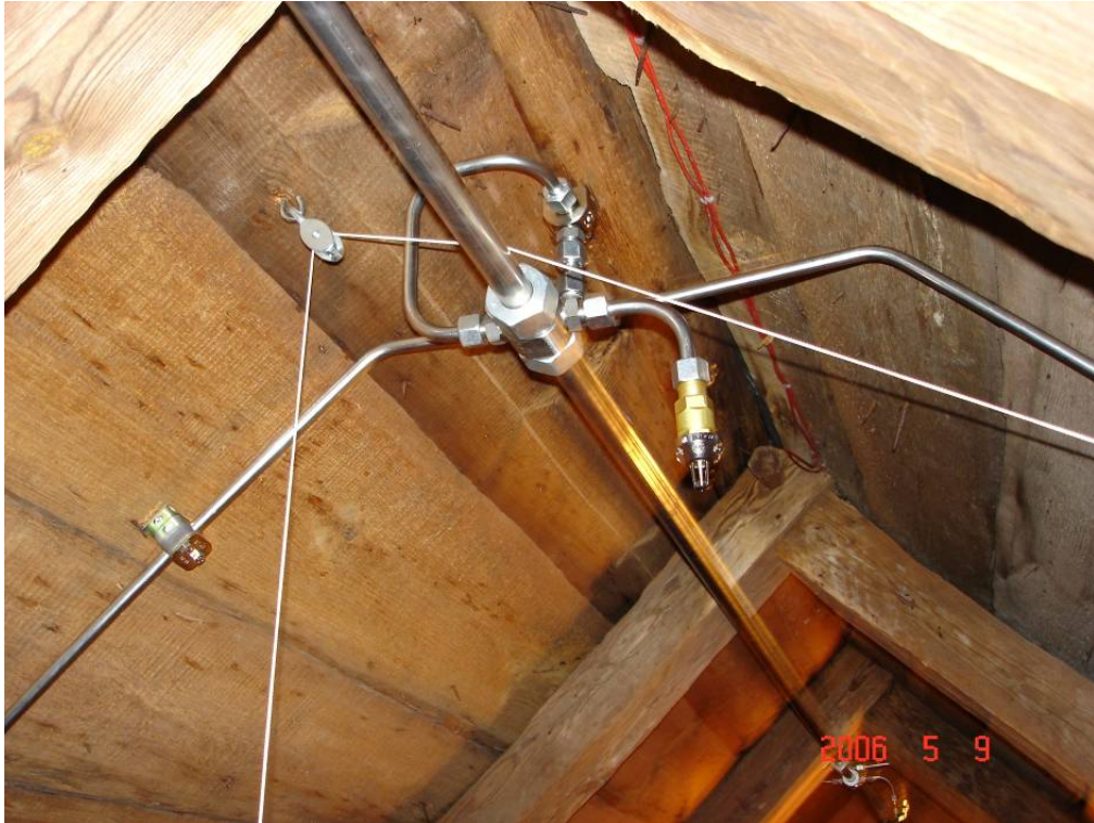
Installation of the high-pressure system inside the attic of the church. The activation of a group release valve (at the top) activates one nozzle on either of the vertical branch lines. In addition, a separate, automatic, pendent nozzle may activate independent of the group release valve.
