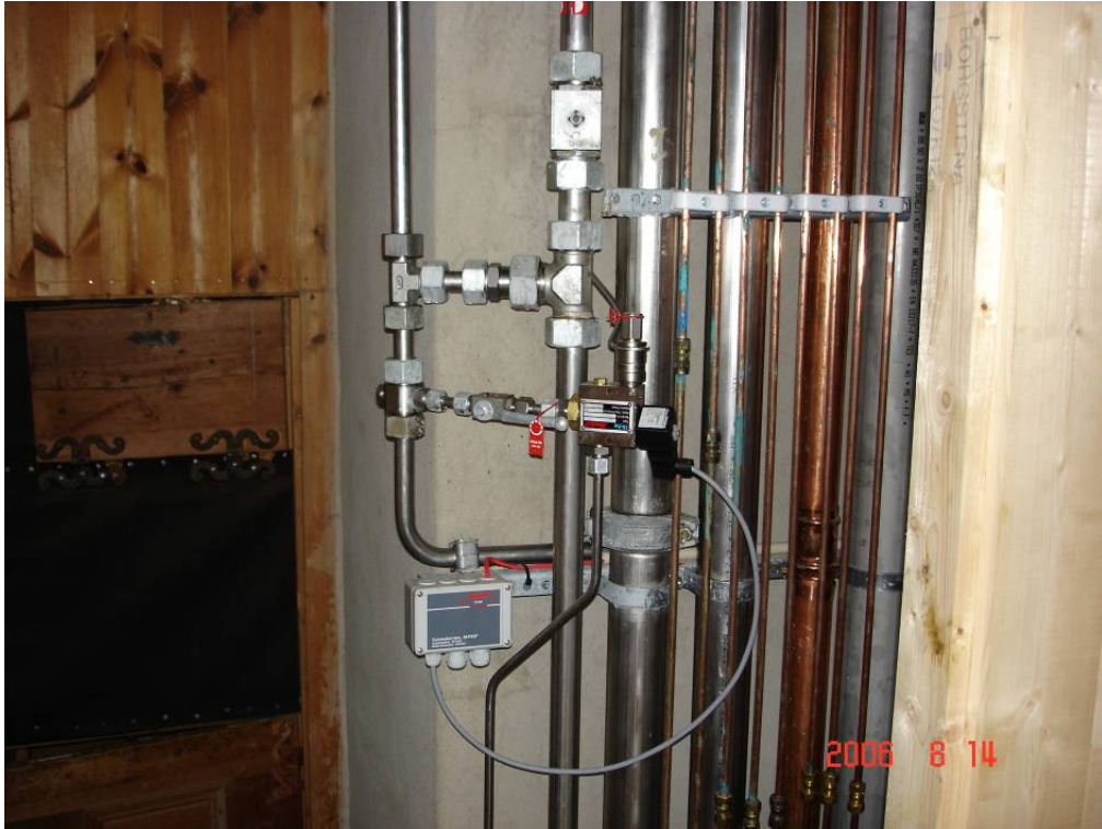
The section valve for the high-pressure water mist system.
