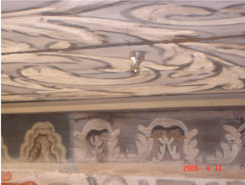
Close-up photo of one of the high-pressure water mist nozzles at the ceiling.
