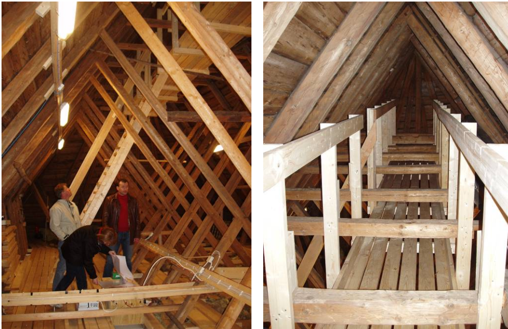
Figure 9 Permanent working platforms inside the attic of Fröskog church. The platform flooring at the top level was built under the beams, to allow full standing height. Photo: Jan G Andersson.
