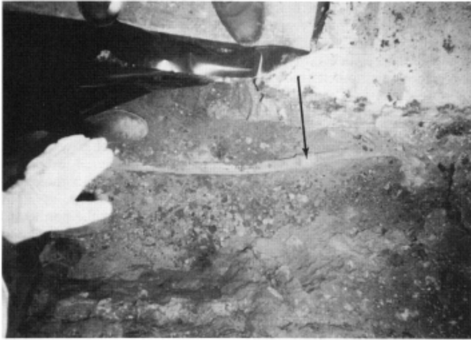
Figure 5. Location of Crack in Plastic Gas Line to Chicken Kingdom.
