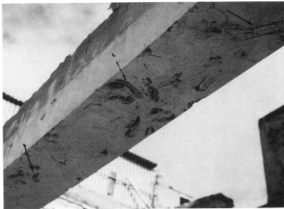
Figure 9. Shoe Sole Imprints on Bottom of Beam in Basement of HV Building.
