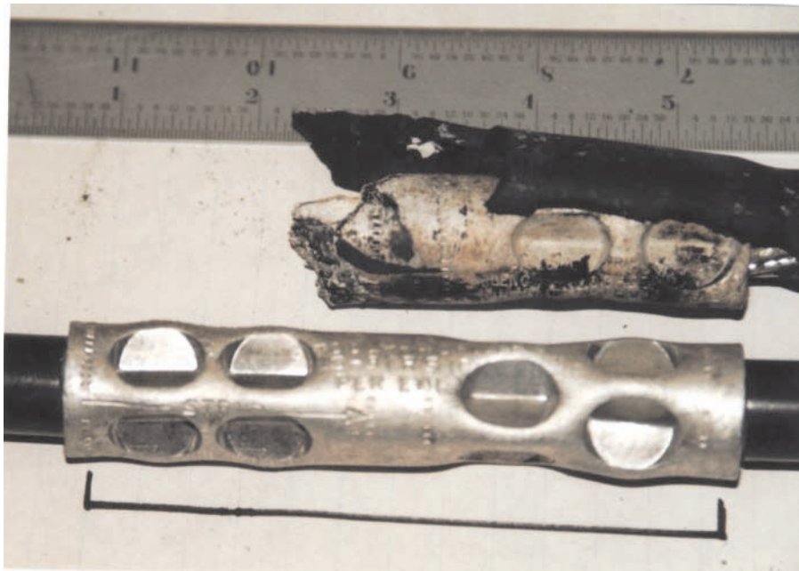
Figure 5. Top: An aluminum crimp connector that was attached to one of the burned electrical cables found in proximity to the damaged natural gas pipeline. Bottom: An exemplar crimp connector (without its cold-shrink insulation).
