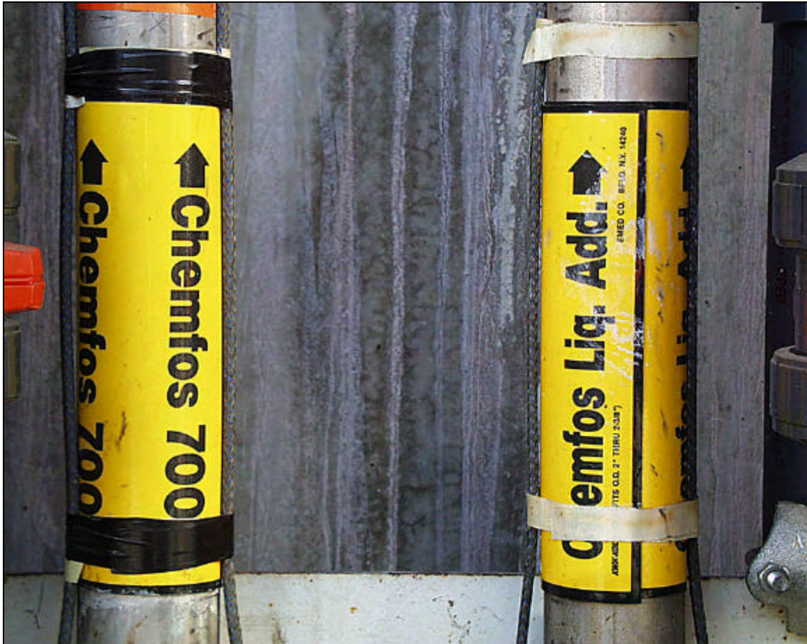
Figure 3. Close-up view of the correct transfer coupler (left) and the coupler to which the transfer hose was inadvertently attached (right)
