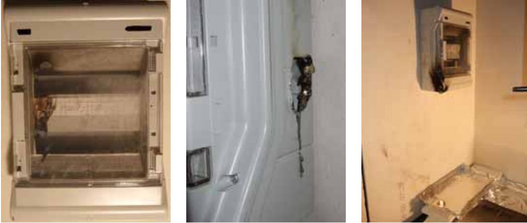
Figure 1-35: Damage done to the enclosure after application of the small premixed flame to position 1, 5 and 7.
