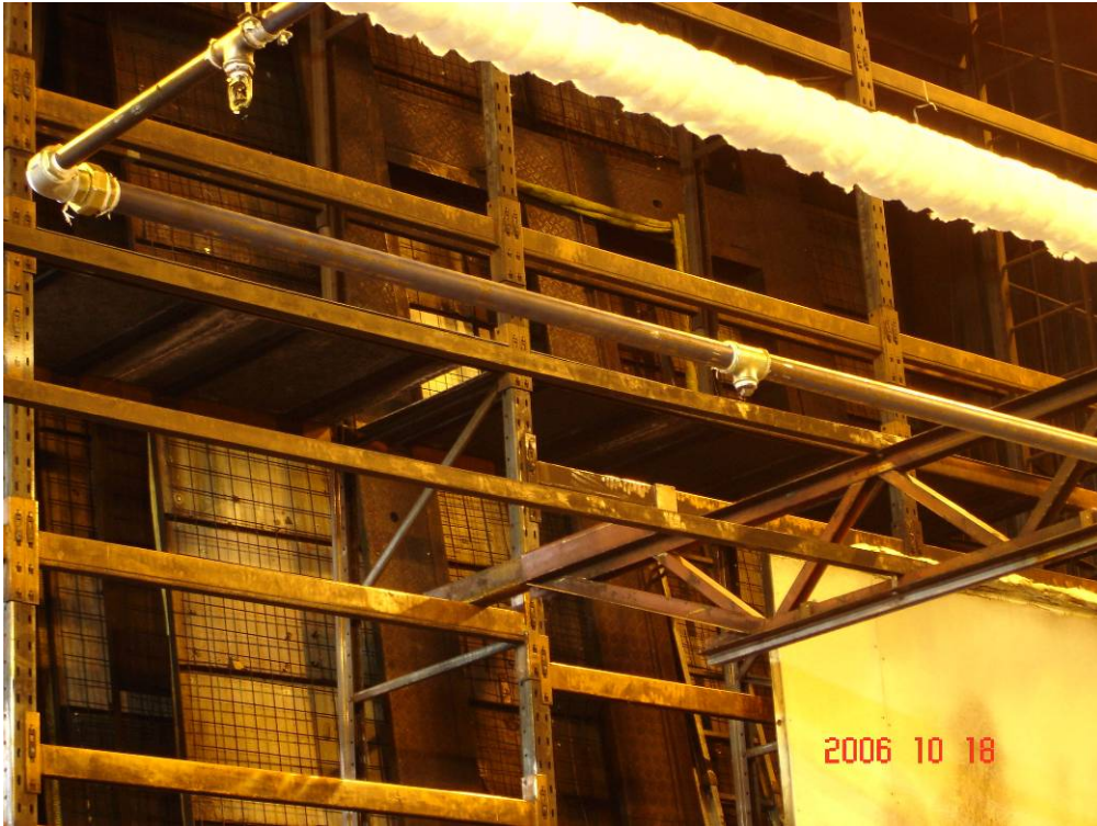
Photo 3 The system pipe-work, which was attached to a framework construction that partly were fire insulated.
