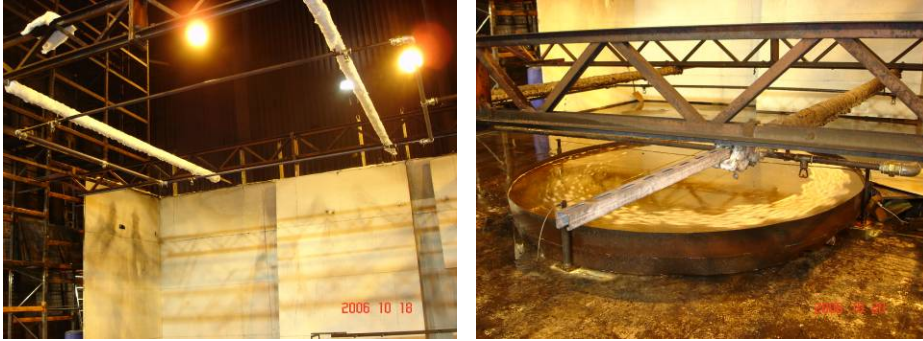
Figure 3 The system pipe-work when positioned at the 'high' elevation (left hand photo) and at the 'low' elevation above the pool fire tray.
