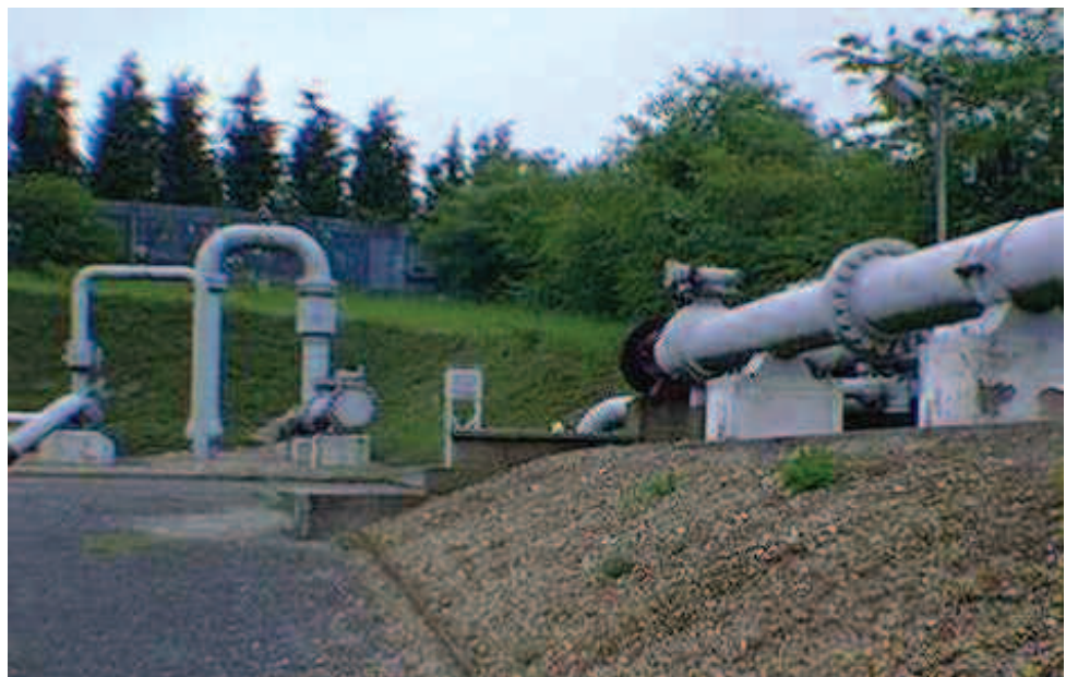
Figure 3 Surface pipelines within an oil fuel depot
