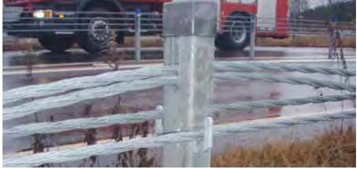
Wire-rope barrier Gunnebo.
