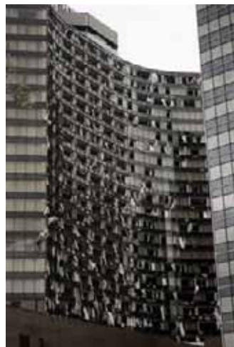
Hyatt Hotel New Orleans nearly all windows blown out
