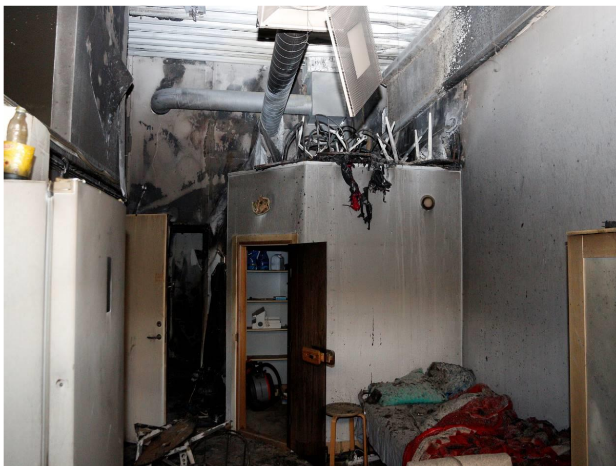
Personalutrymme, brand ovan undertak.
