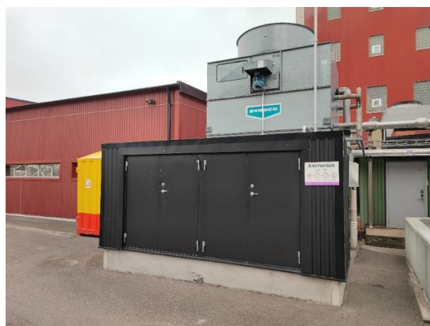
Figur 4 - Inbyggd ammoniaktank (receiver). Bakom receivern syns kondensorn.
