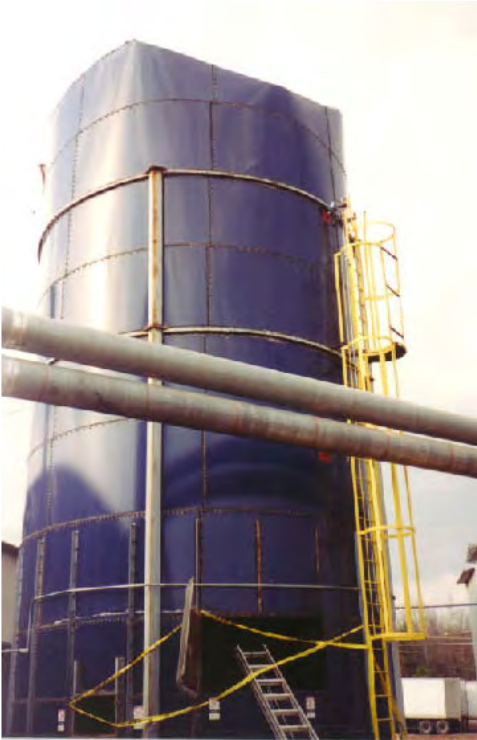
Photo 2. Access plate, origin of explosion
