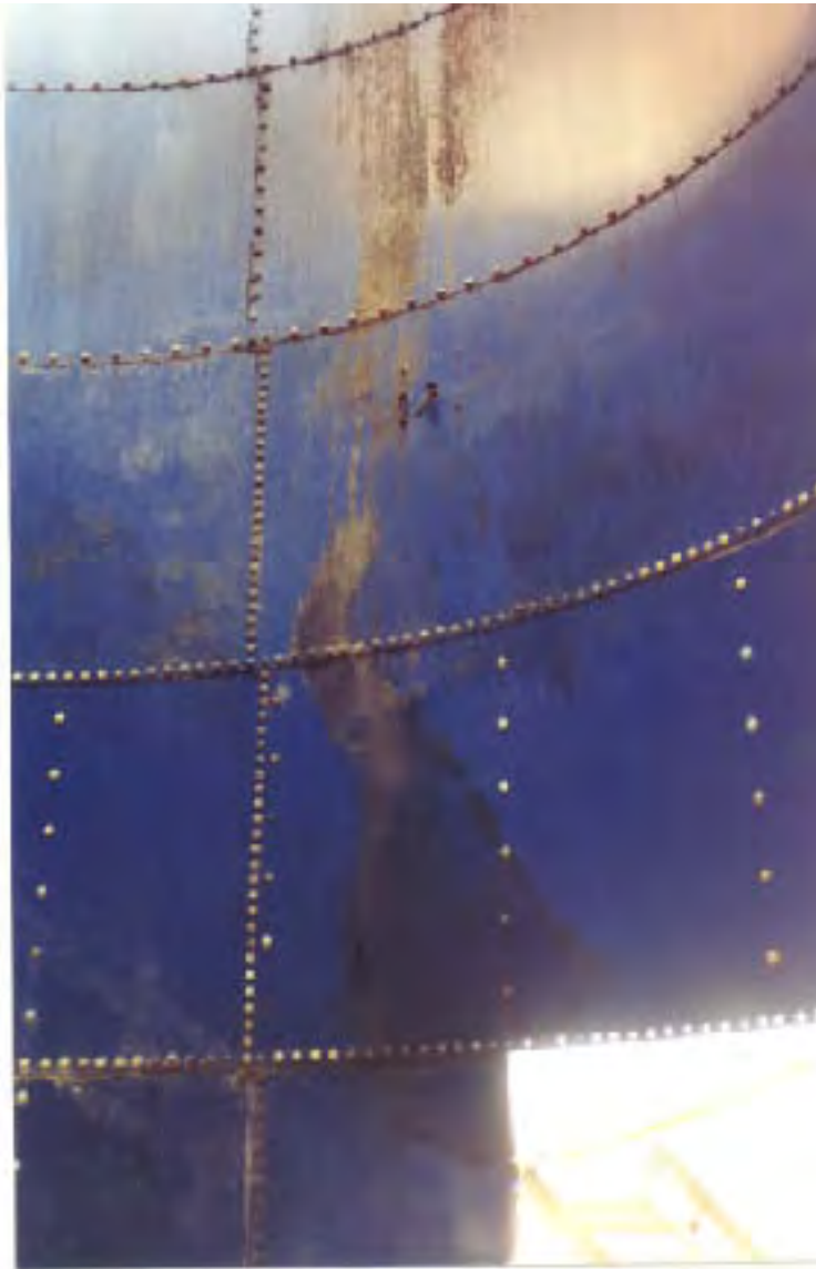
Photo 8. View from inside silo showing burned-out areas in relation to access panel (origin of explosion)
