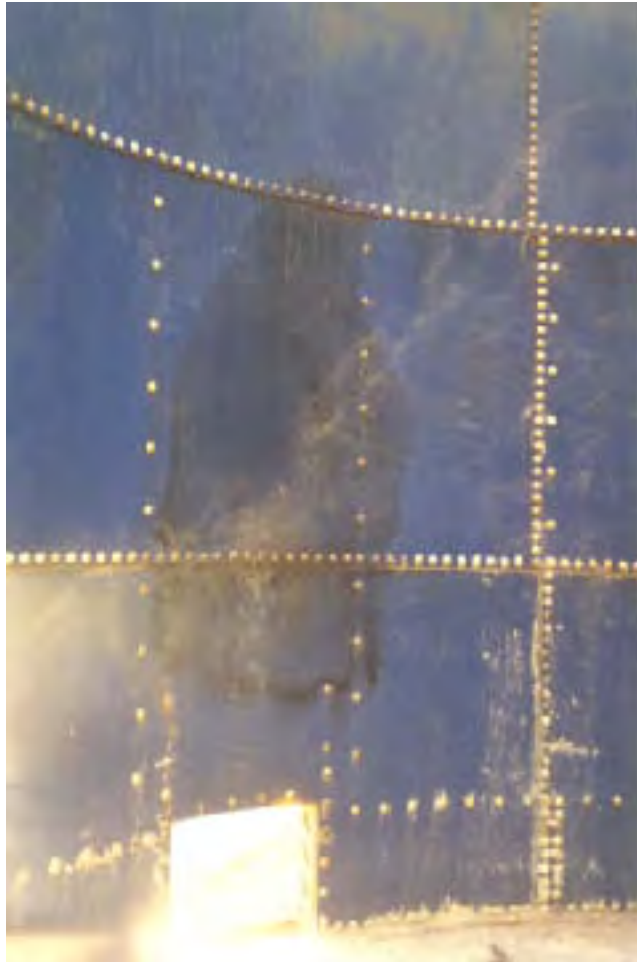
Photo 5. Smaller access panel indicating burning in stack above 2'x2' access panel (panel removed for post-fire investigation)
