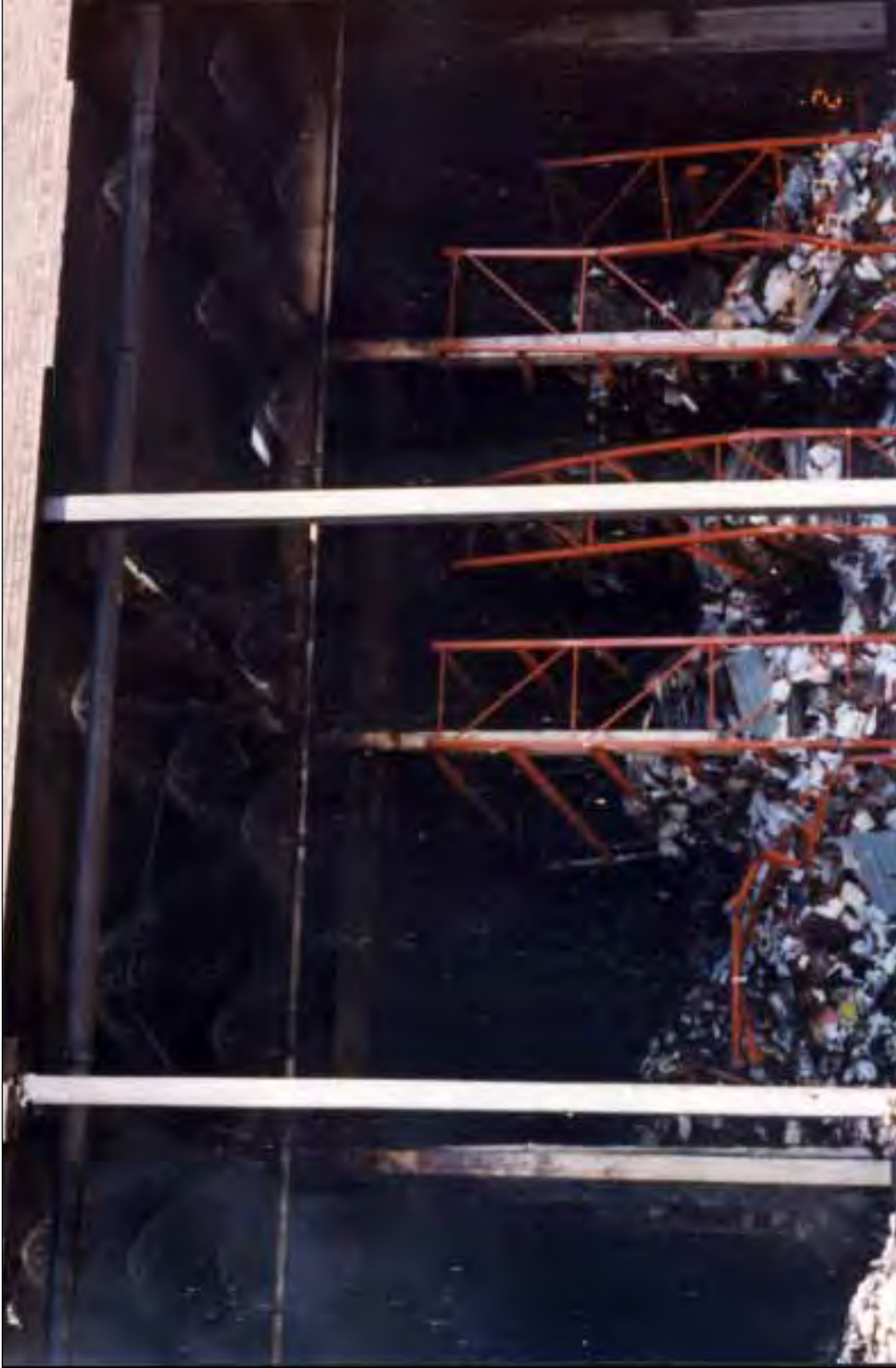
3. Racks and operating overhead automatic sprinklers near the northwest corner of Building III. Complete and partial collapse of the storage racks, shelves, and contents.
