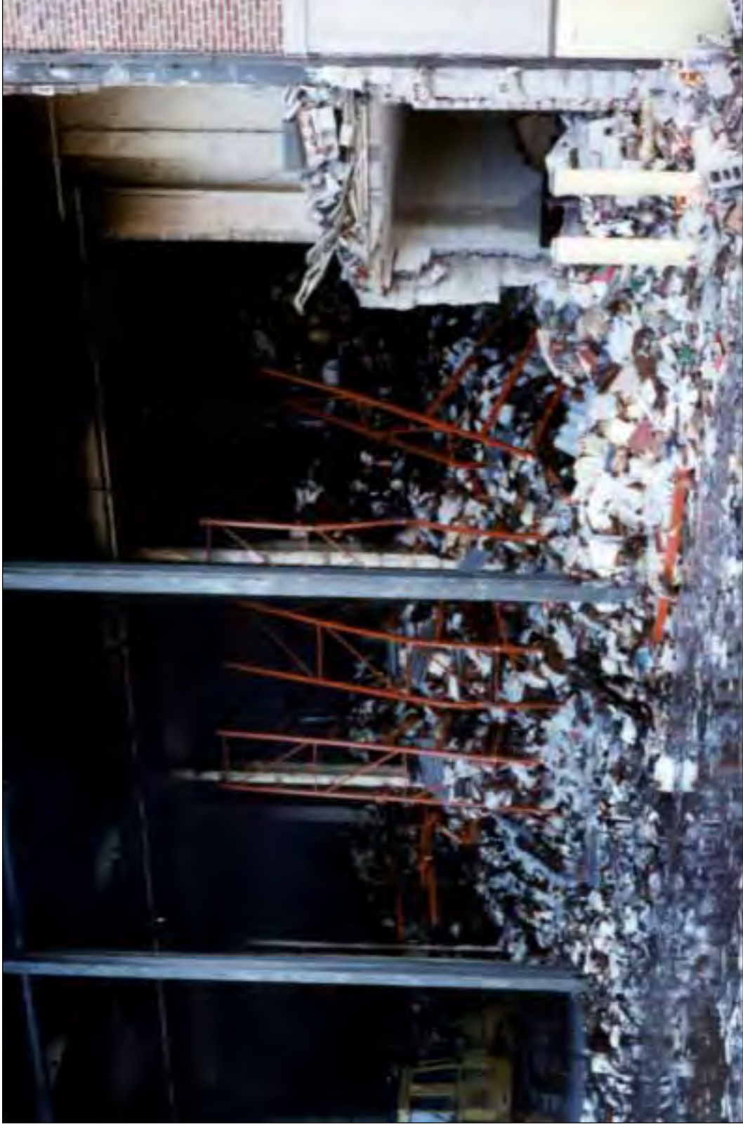
2. Typical of the rack collapse, record box failure, and documents filling the aisles. The brick-faced, hollow concrete block front wall was removed on the night of the fire.
