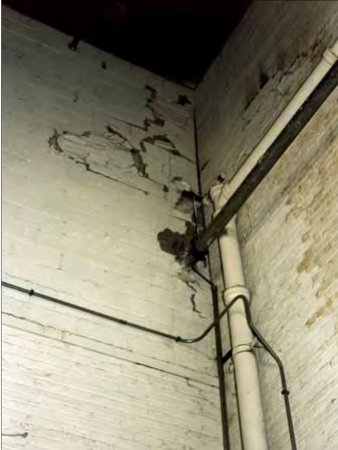
7. Masonary wall damage in Building II, north of the fire building, due to expansion of the fire wall between buildings. This corner is the southeast corner of Space 6.
