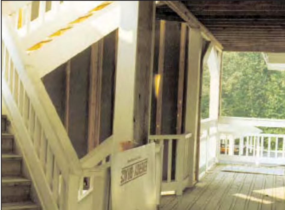
10. The stairway and exterior walkways used throughout the building. Note the gaps in the walkway to allow water to drain and the piece of thin exterior sheathing leaning against the stairway.
