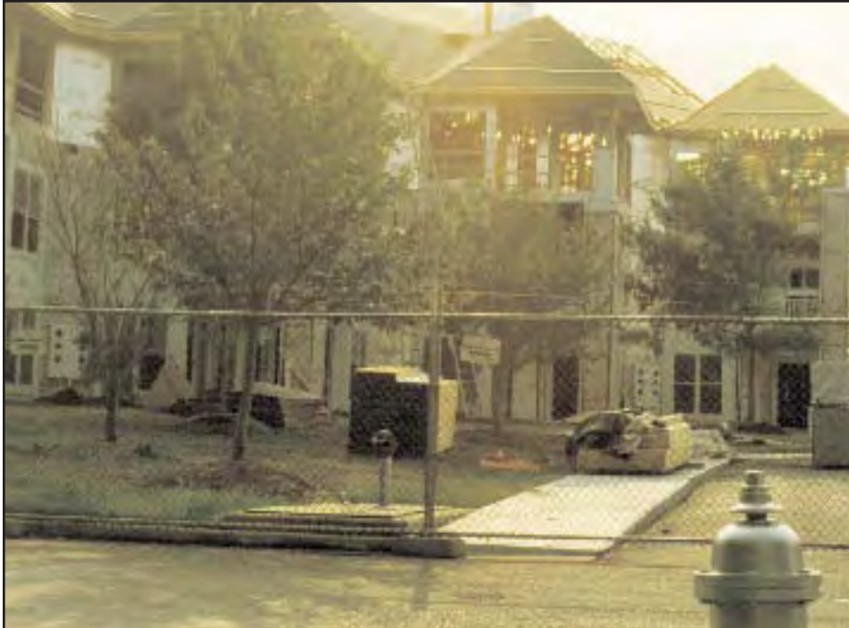
6. Fire hydrant and core siamese connection used by Engine 54 on arrival. Repairs and reconstruction are being made to the front wing; this side is the patio/balcony for each apartment.
