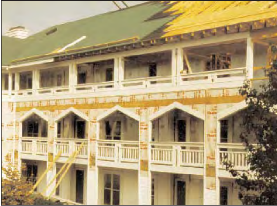
9. The exterior walkways in Sector D, with the stairway located at the left edge of the photograph. The core is out of the picture to the right.
