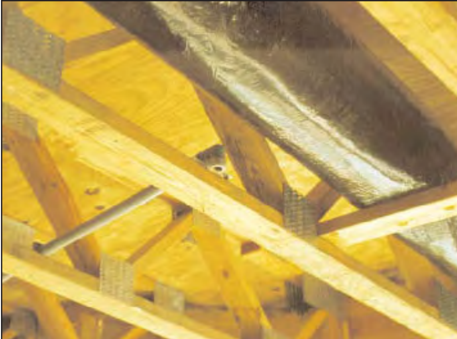
12. The parallel cord wood floor trusses used in the original construction and a polybutylene automatic sprinkler line.
