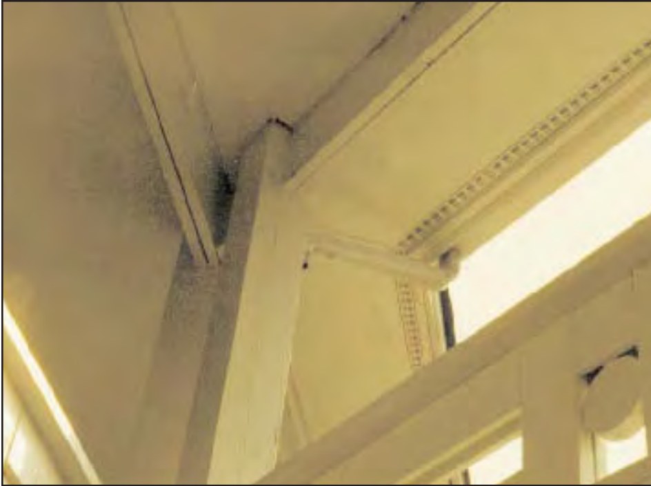
11. Typical eave line vents installed around the perimeter of the building. The fire is believed to have entered the attic through these vents.
