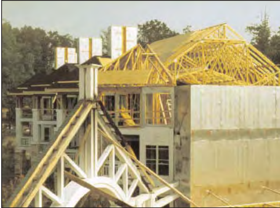
7. The remains of the front archway and the repairs and reconstruction underway for the wing in Photograph 6. The attic trusses and exterior sheathing materials are illustrated.
