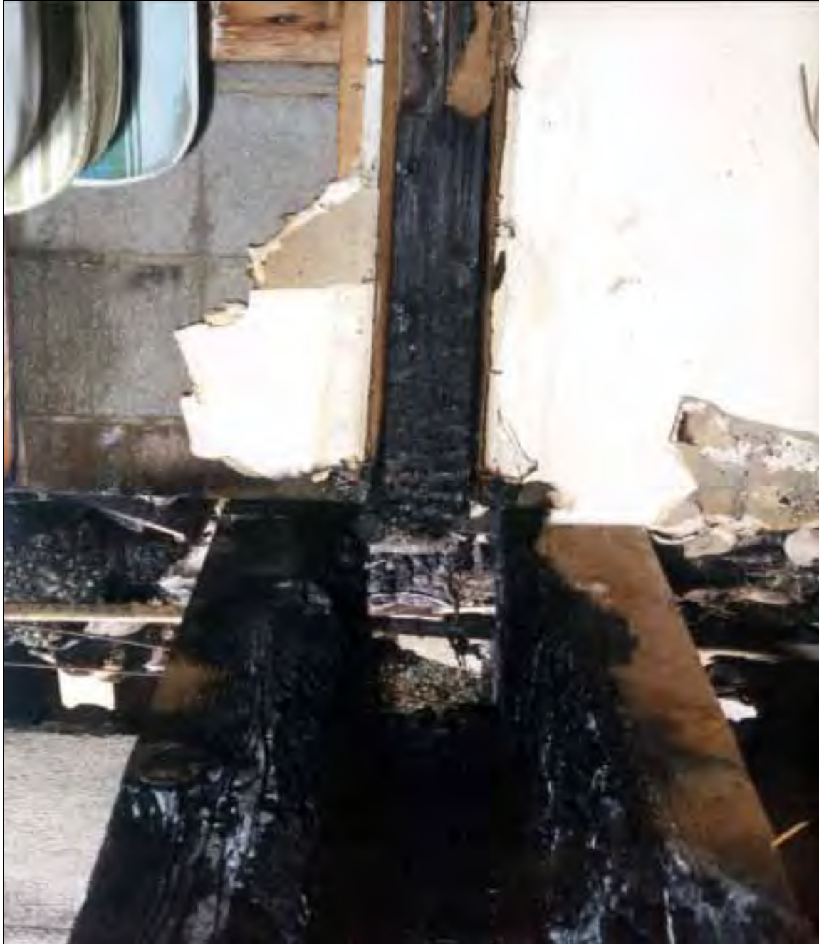
9. A separation wall between 100 level guest rooms that was burned from the inside out. The parallel wood beams formed the top of the wall and the communication to the utility chase is at the back.
