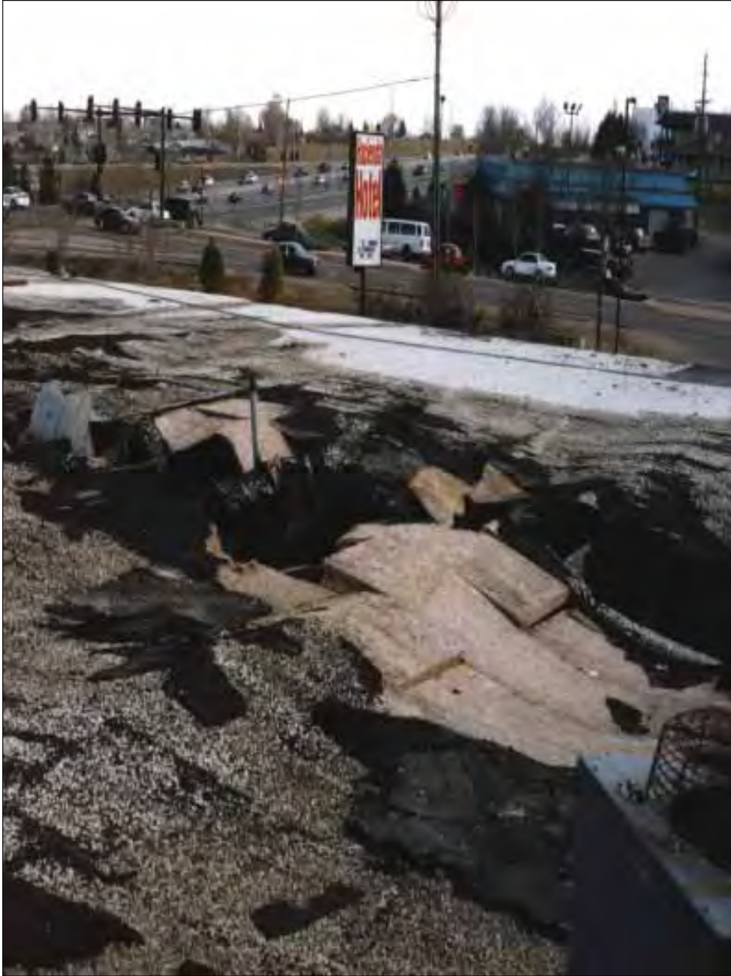
6. Roof over the front wing. The collapsed area is above the utility chase. The roof construction of Tectum board, built-up roofing, and gravel topping is illustrated.
