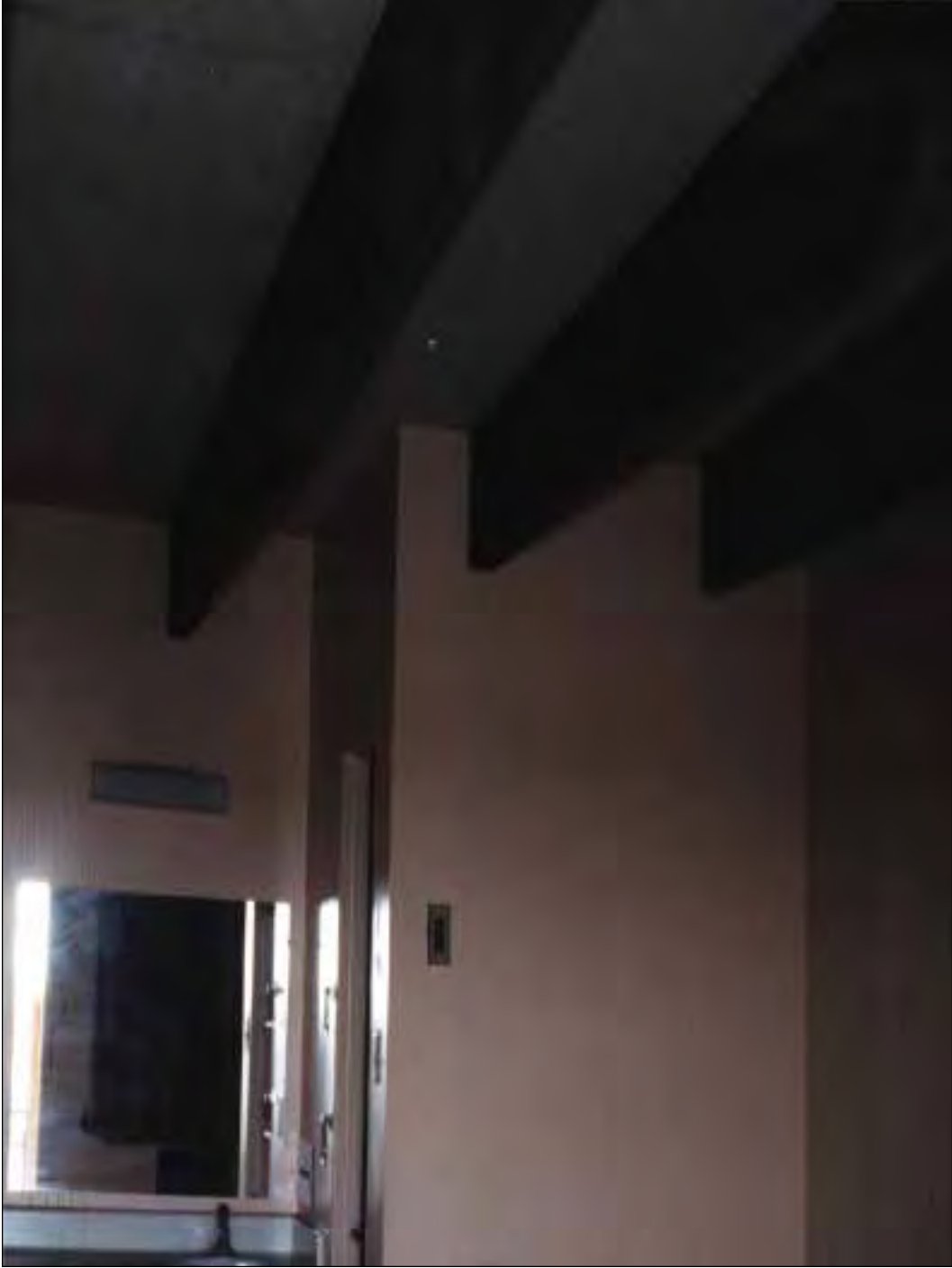
4. Typical guest room ceiling, bathroom, and sink on the utility chase wall.
