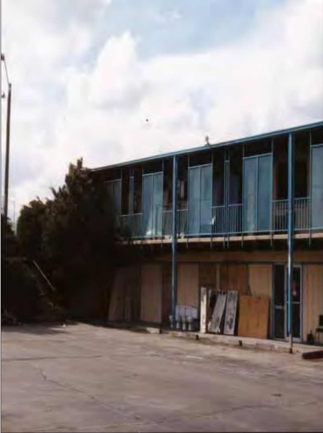
1. Southwest corner of the front wing looking northwest. The 100 level commercial and offices and the 200 level guest rooms are shown. The pine tree shields the entrance to the stairway and storage closet which was the point of origin.
