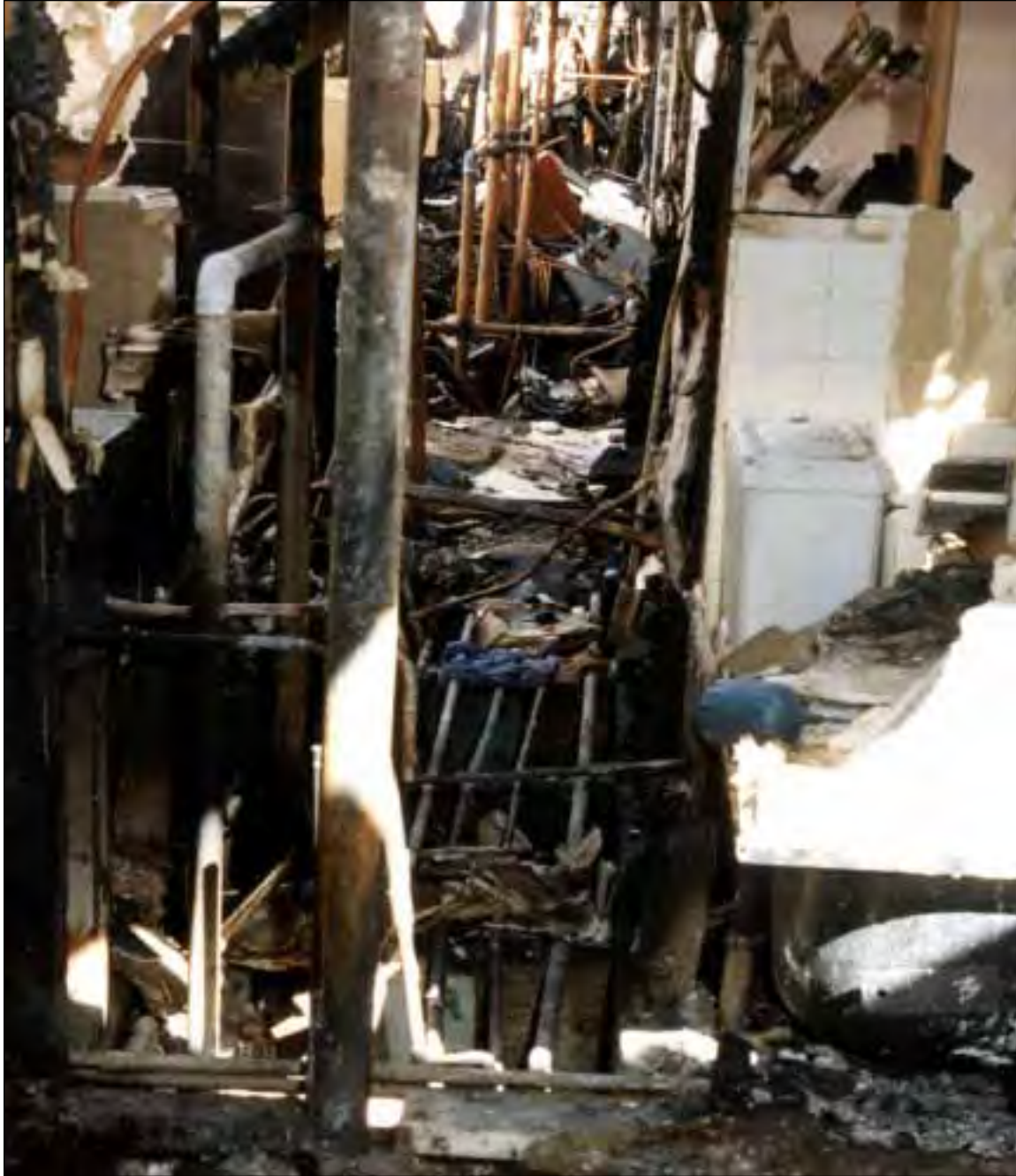
7. The west end of the utility chase in the front wing. Room 222 is to the left and Room 211 to the right. The second floor utility chase walls were burned away.
