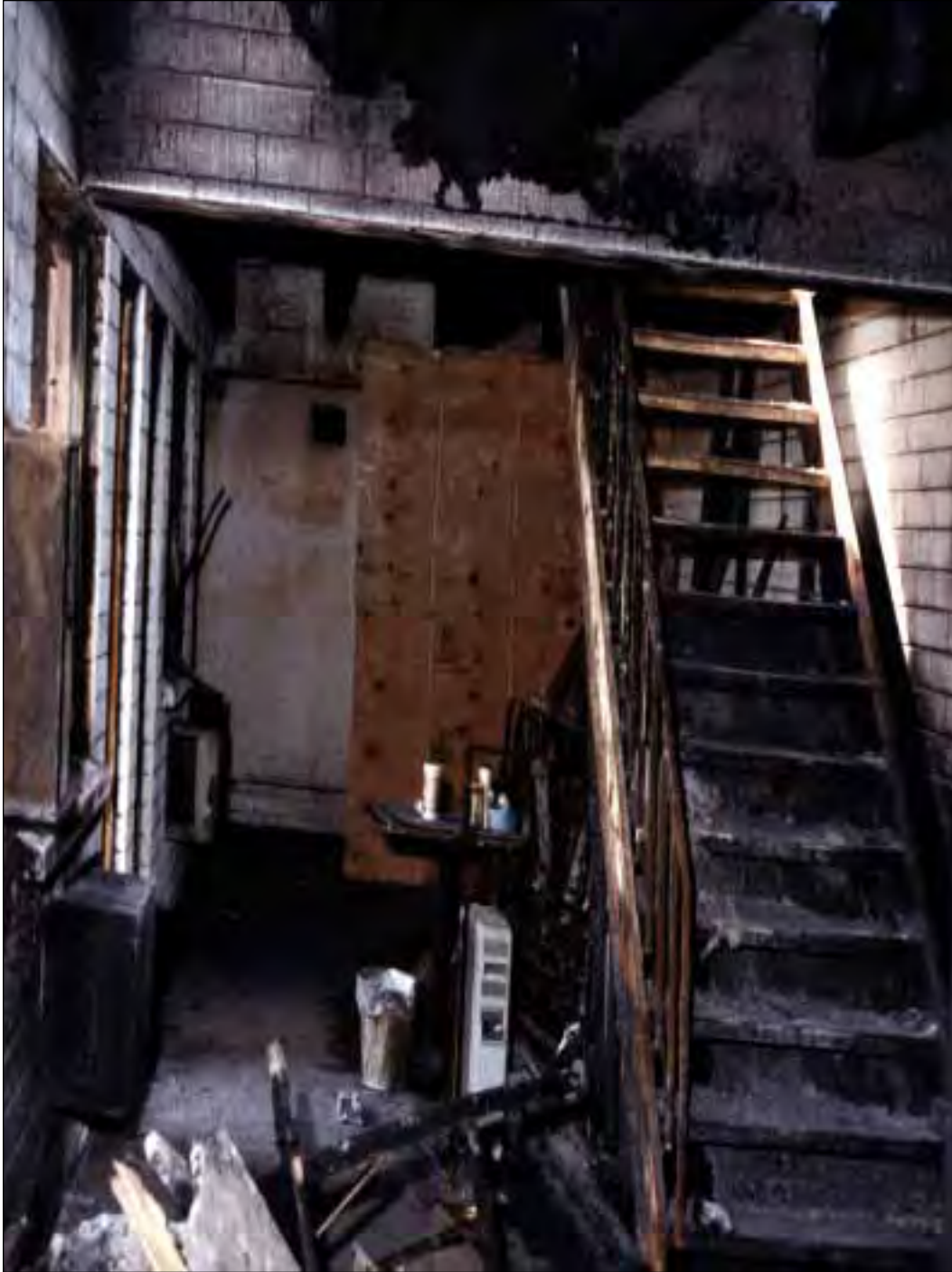
8. The 200 level breezeway area outside of Rooms 220 to 222 looking west. The open stairway to the 300 level is on the right. Under the stairs is another storage room whose wood stud and gypsum board walls were destroyed by the fire.
