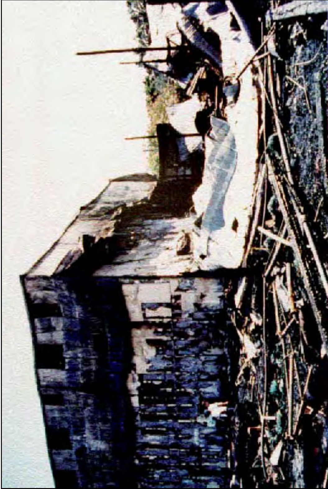
2. View looking east from Manufacturing Building (Building A) towards the destroyed Office Building (Building C).
