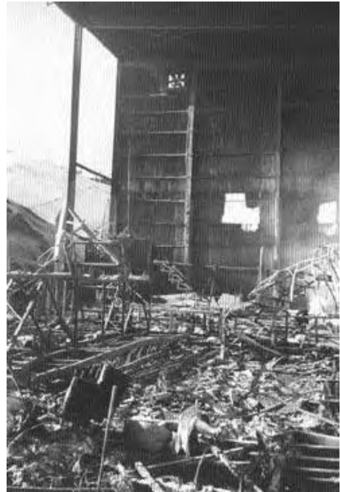
This is the skeleton of the 40 x 40 foot hallway which allowed the fire to communicate to the prop assembly and maintenance buildings.
