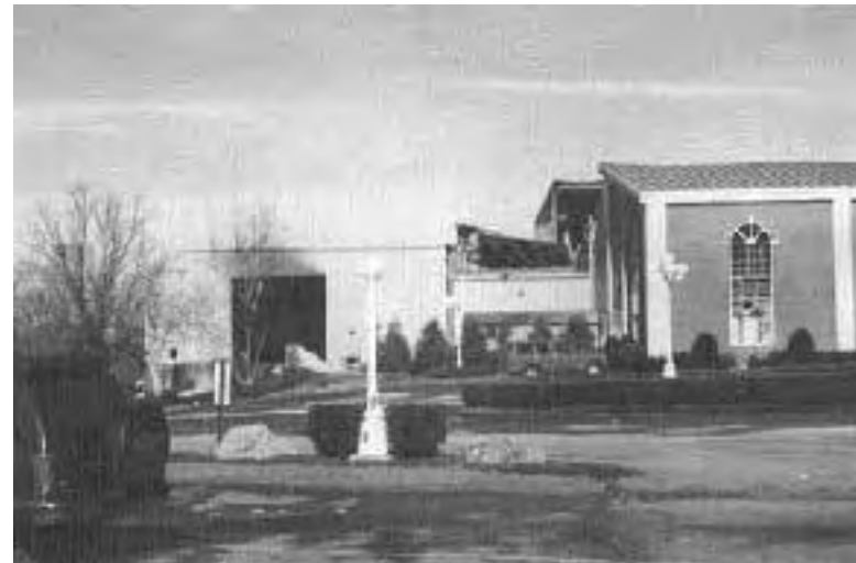
This picture is taken from the front, looking toward side two of the building, which shows the auditorium roof and side stage roof collapse.
