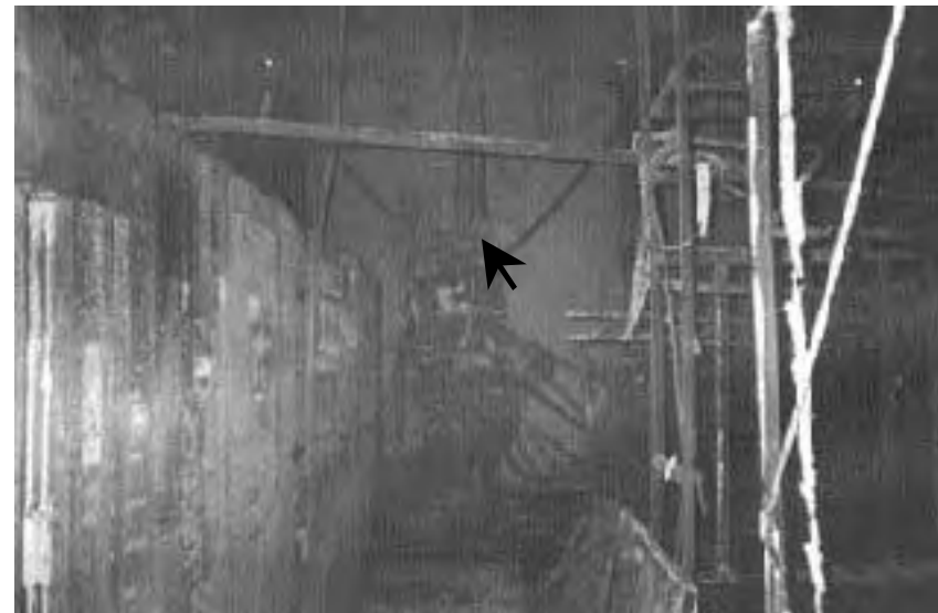
Remains of some scenery prop frames which were obstructions to hose line advancement and locating the fire. Also visible hanging from the ceiling is the wire mesh used to support the spray-on fire protection which was damaged during the floor renovation.
