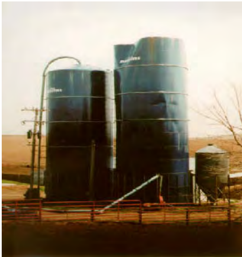
Deformity of silo shell due to explosion
