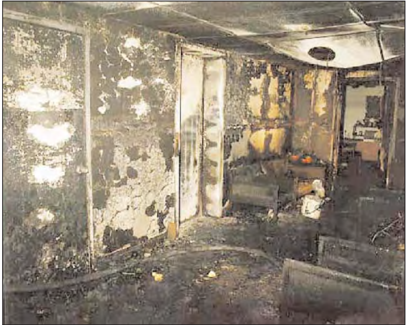
3. View of office waiting area on second floor from the SE stairway door.
