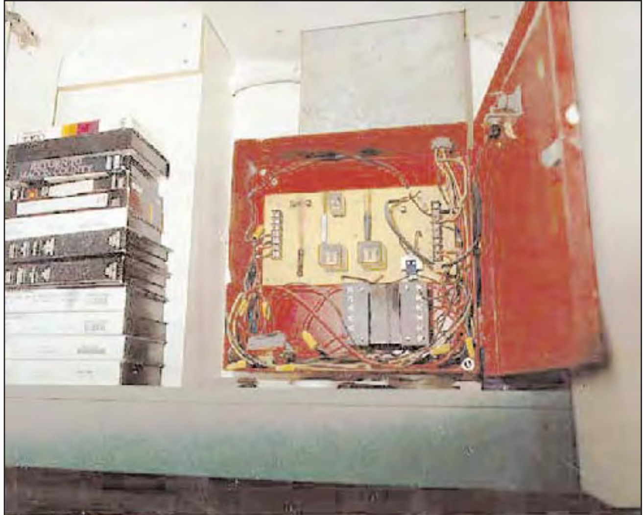
6. Fire alarm control panel. The panel was located inside a cabinet in the first floor front office. Note the on/off switch in the bottom left hand corner of the box.
