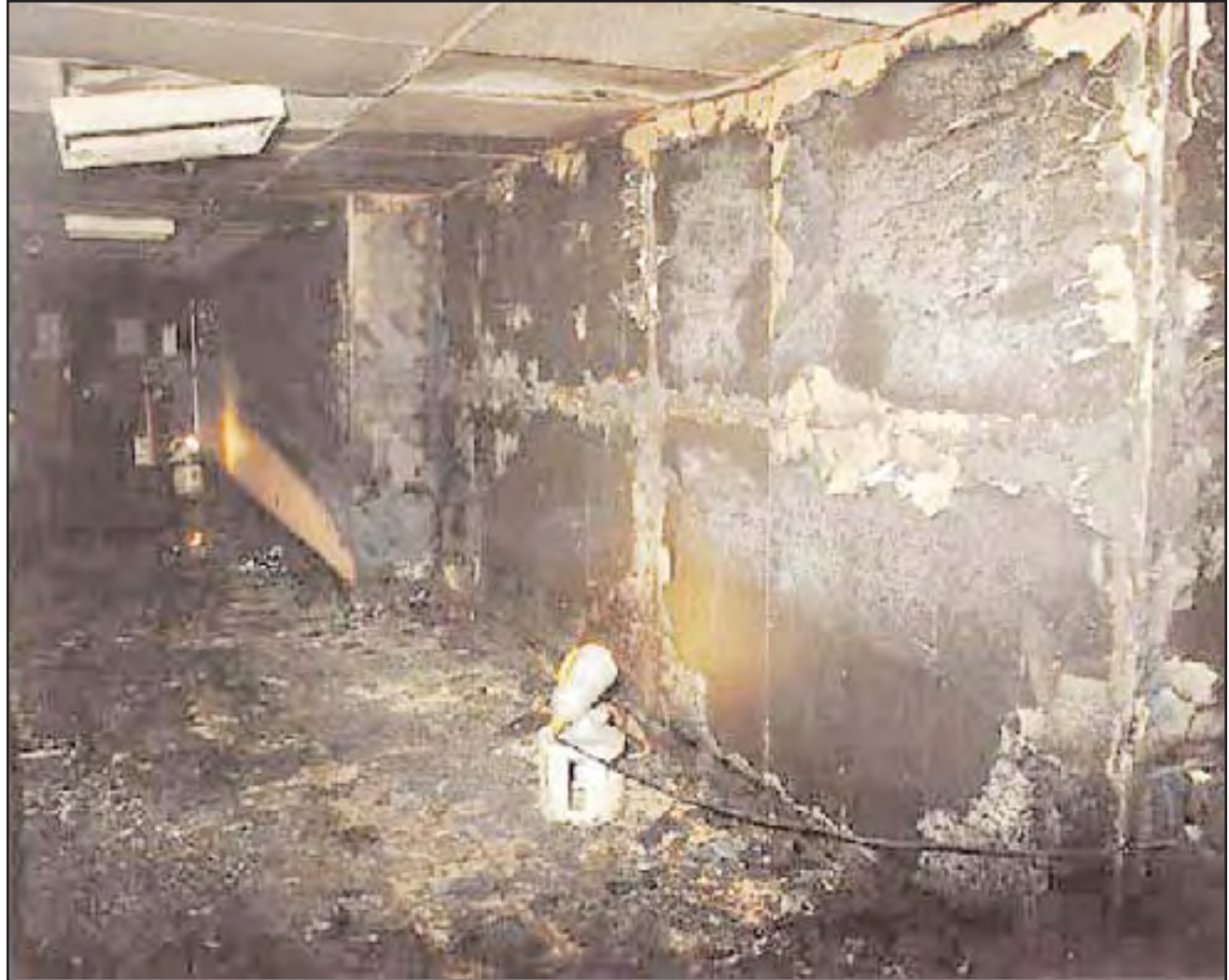
4. First view of hallway leading from office waiting area to residential areas of the second floor.
