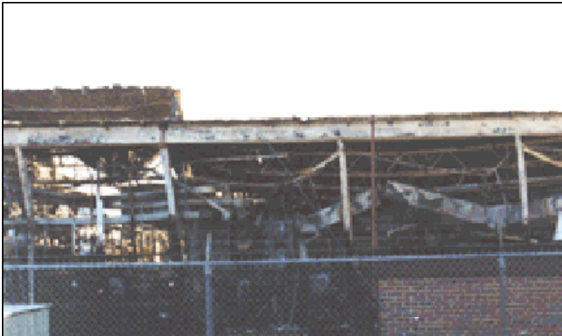
14. The east fire pump house and a view into the building showing some of the manufacturing equipment and ductwork. The west side of the heat transfer fluid boiler in photographs 4 and 13 is on the left edge of the photograph.
