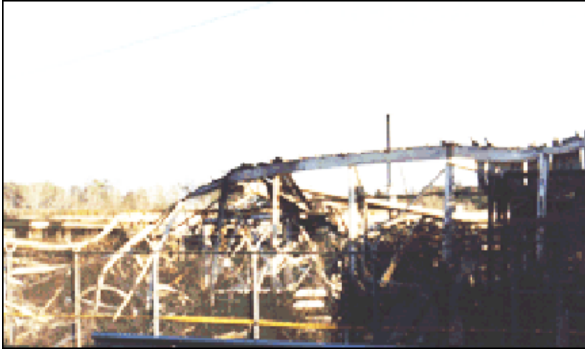
13. Some of the same area in photograph 4 but from a different angle and after the fire. In the bottom right hand corner is one of the heat transfer fluid boilers.
