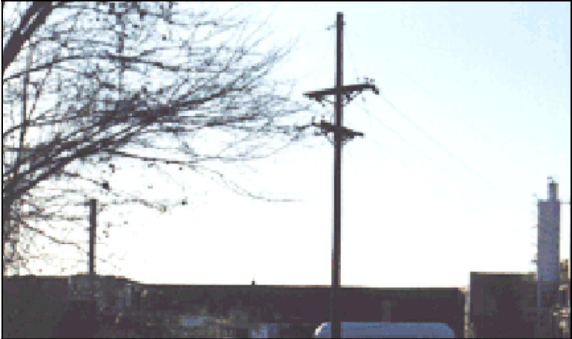
11. Several days after the fire, the northeast corner of the complex. The LP-gas storage tanks, raw material storage silos, and heat transfer fluid boilers and support equipment are shown. Taken from Swift Street looking west.
