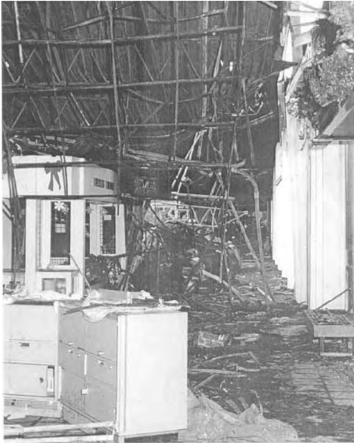
Photograph 6. Moving further east in the covered mall, the counters in the foreground are also in Photograph 3. This area is where the metal roof began a partial collapse. The goods in the kiosks were either stored before the fire or removed prior to the picture.
