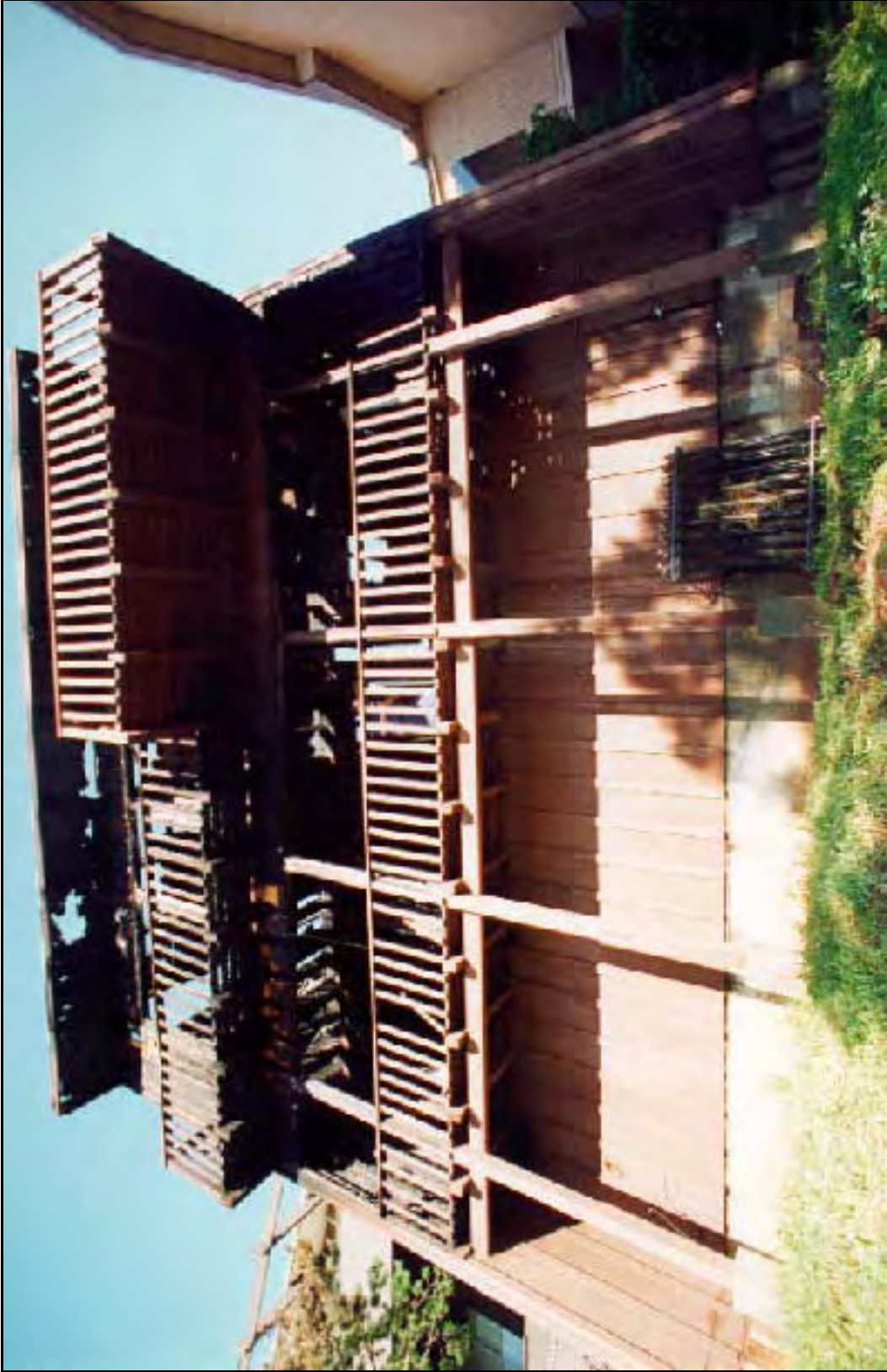
PHOTOGRAPH 2 The rear of the house as viewed from ground level. The fire started in the wall above the lower deck to the right center of the photograph.
