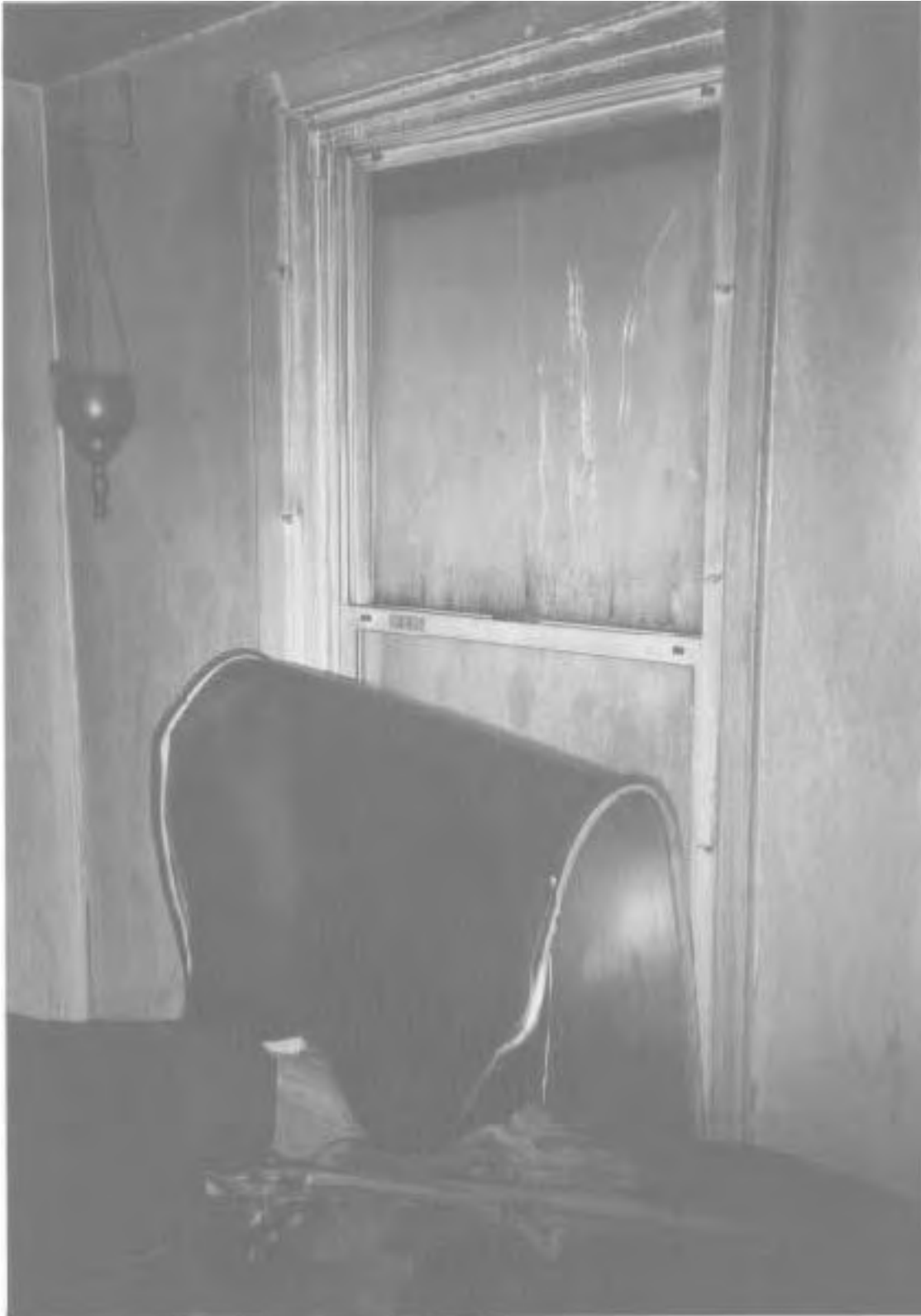
Window in corner of family room showing plastic panel which has partially melted and bent-over due to heat.
