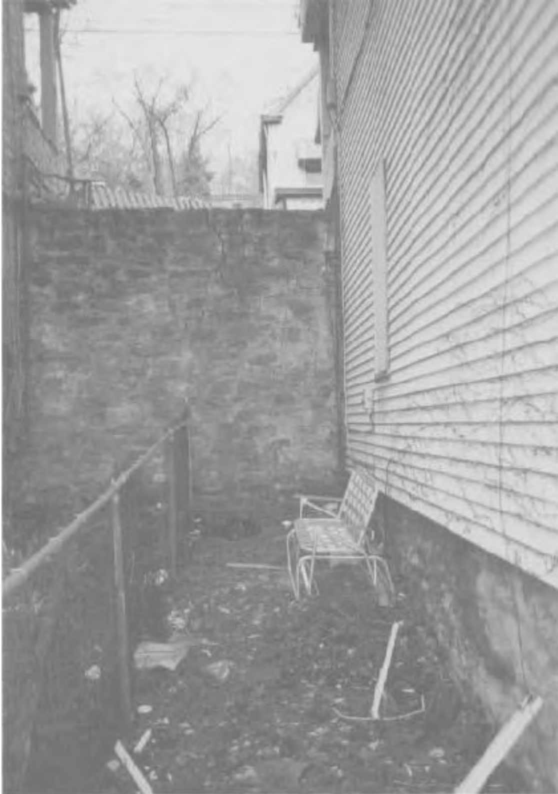
Side yard showing retaining wall and window where firefighters were rescued (above lawn chair.)
