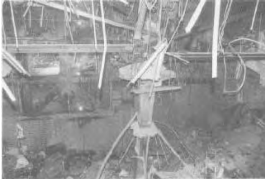
A view of the crater from the B-1 to B-5 levels. Note the steel column. Horizontal supports were destroyed in some cases, but the columns did not give. (Photo courtesy of Port Authority Risk Management.)
