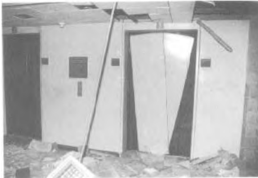
Damaged elevator doors and enclosures on the B-2 level presented a vertical channel for smoke spread into Tower 1. (Photo courtesy of Port Authority Risk Management.)
