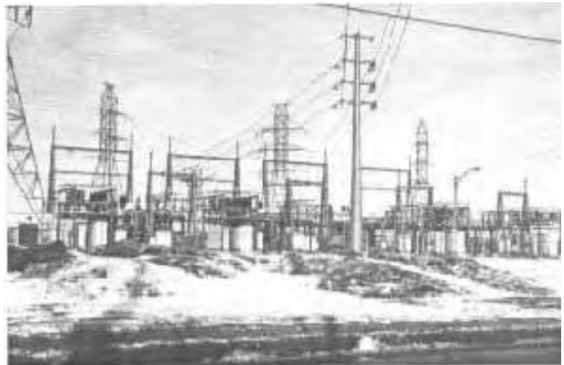
New transmission facilities route power to Du Pont's sodium shop.
