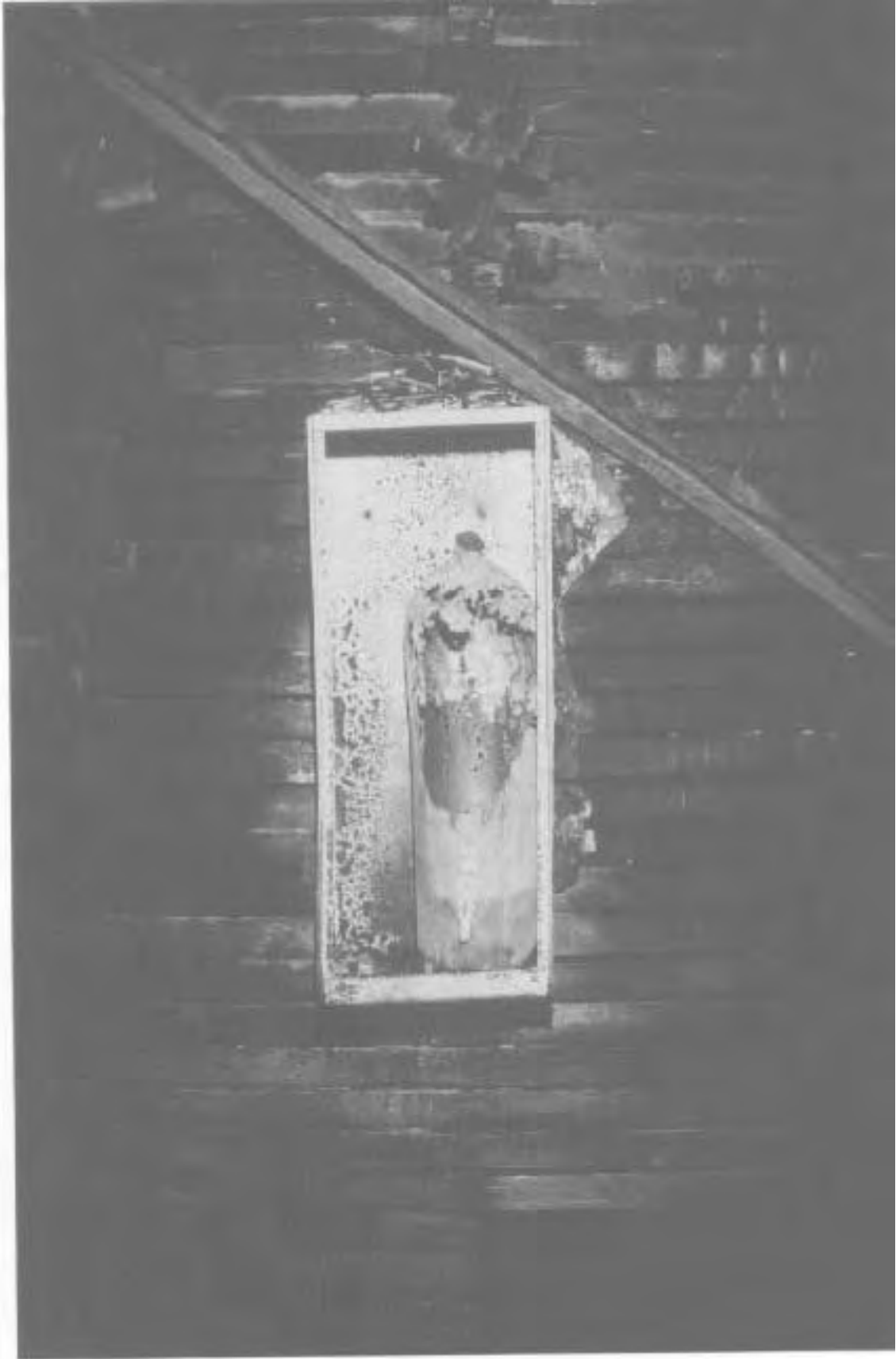
The remains of a melted aluminum fire extinguisher shell in a cabinet on the second floor west side.
