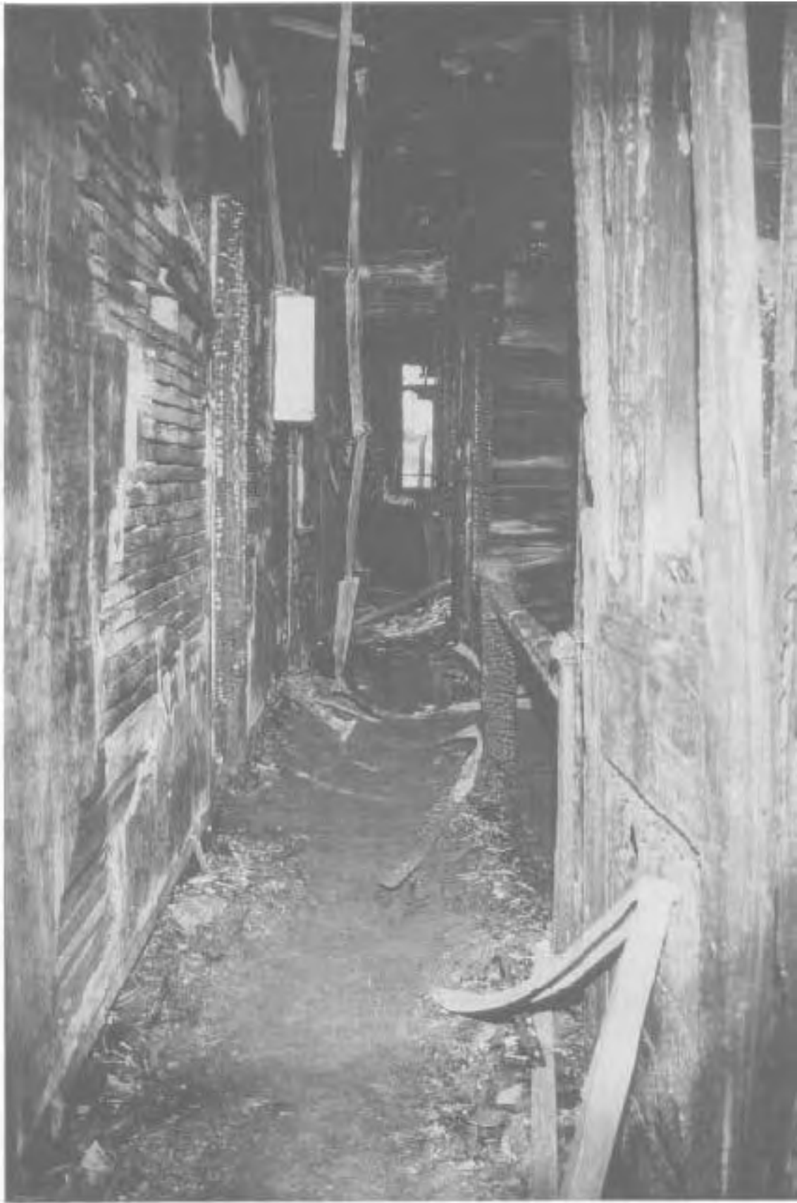
Second floor west corridor looking south shows the heavy fire damage resulting from vertical fire spread via the front stairway.
