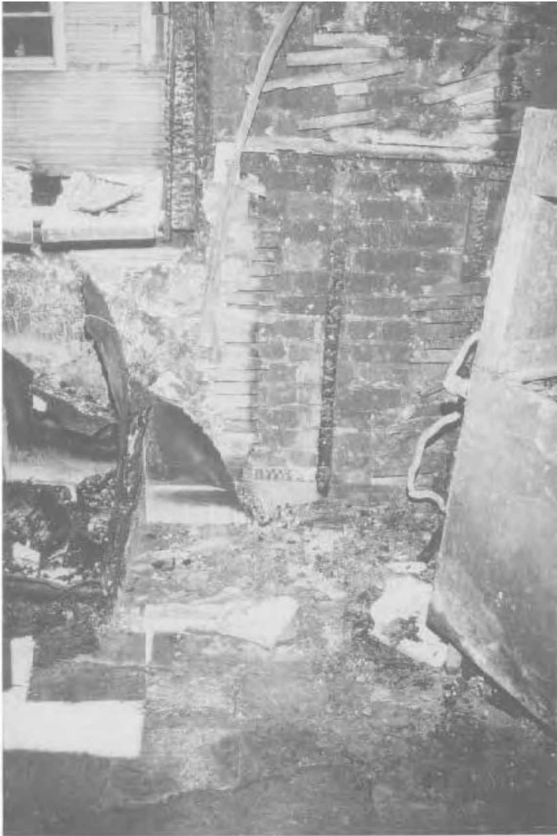
Point of origin in kitchen showing evidence of low burn near the baseboard.
