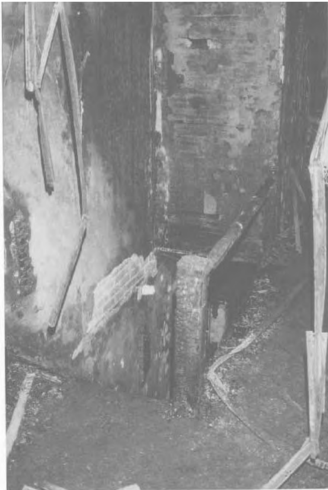
West side rear stairway looking down from second floor. Extensive charring and plaster spalling provide evidence of the fire spread which cutoff access to both the front and rear stairways.
