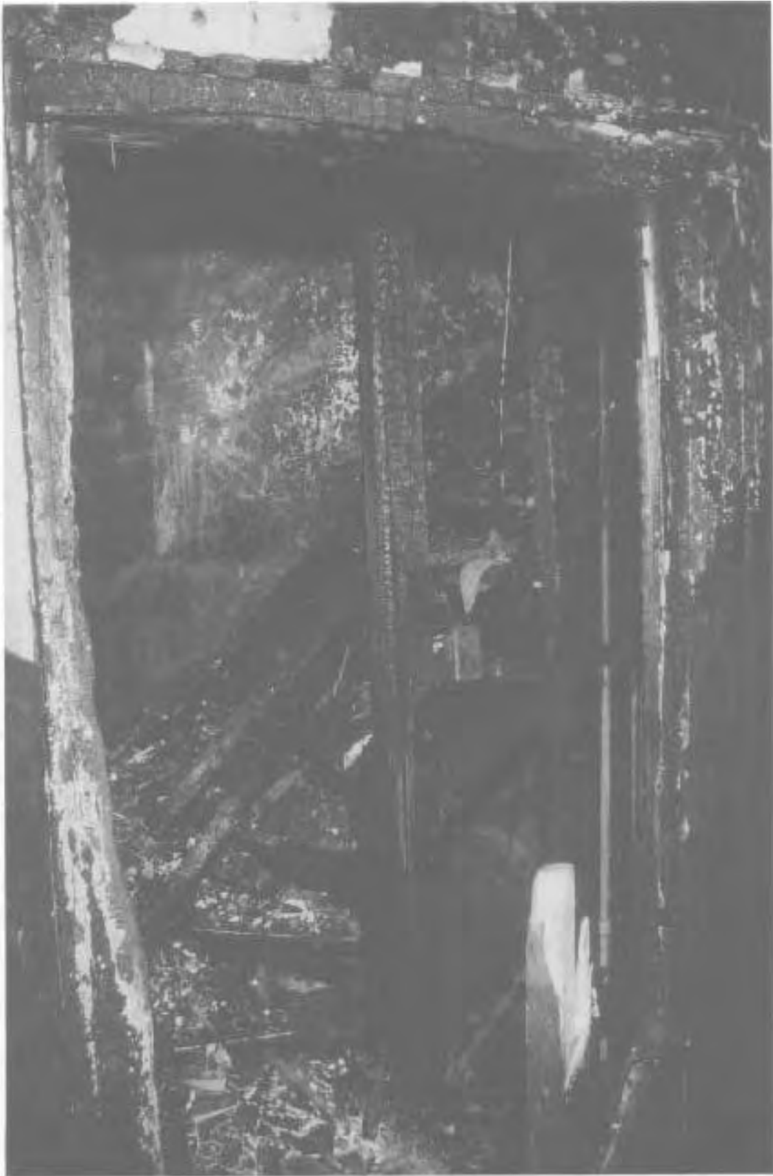
View of west side stairway leading to the third floor. Once again, heavy fire damage to the door lintel and framing indicate that fire spread via this route was extensive.
