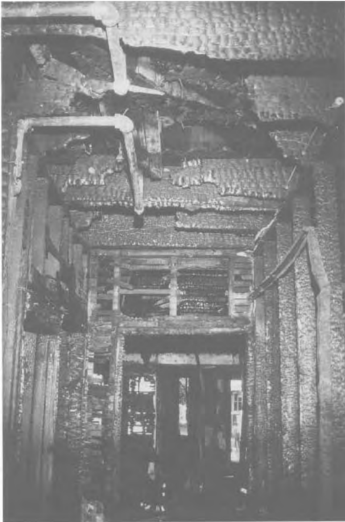
Close-up of fire damage to the ceiling area in rear corridor next to kitchen. Pipe penetrations were one avenue of fire and smoke spread to the second floor.
