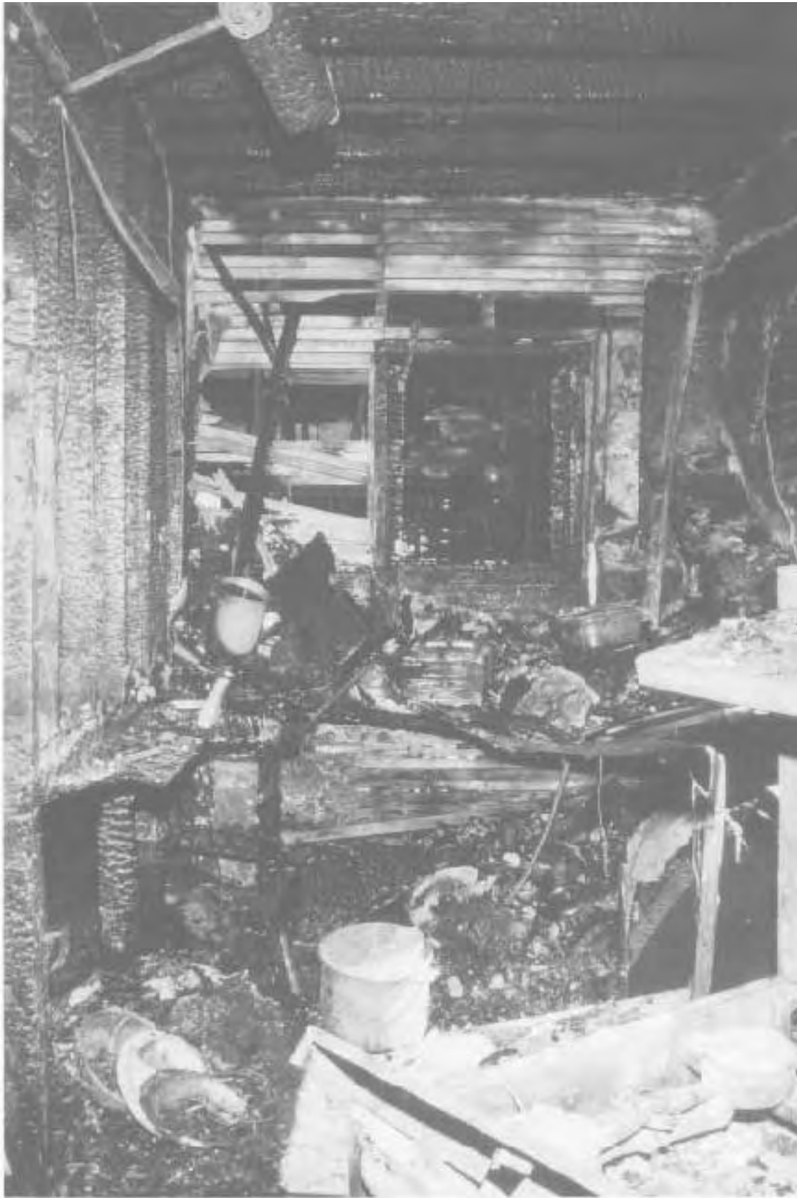
View from the kitchen looking south through the pass-through window into the dining room. The fire was observed through this window by Mr. Fluckes and Mr. Gregory.
