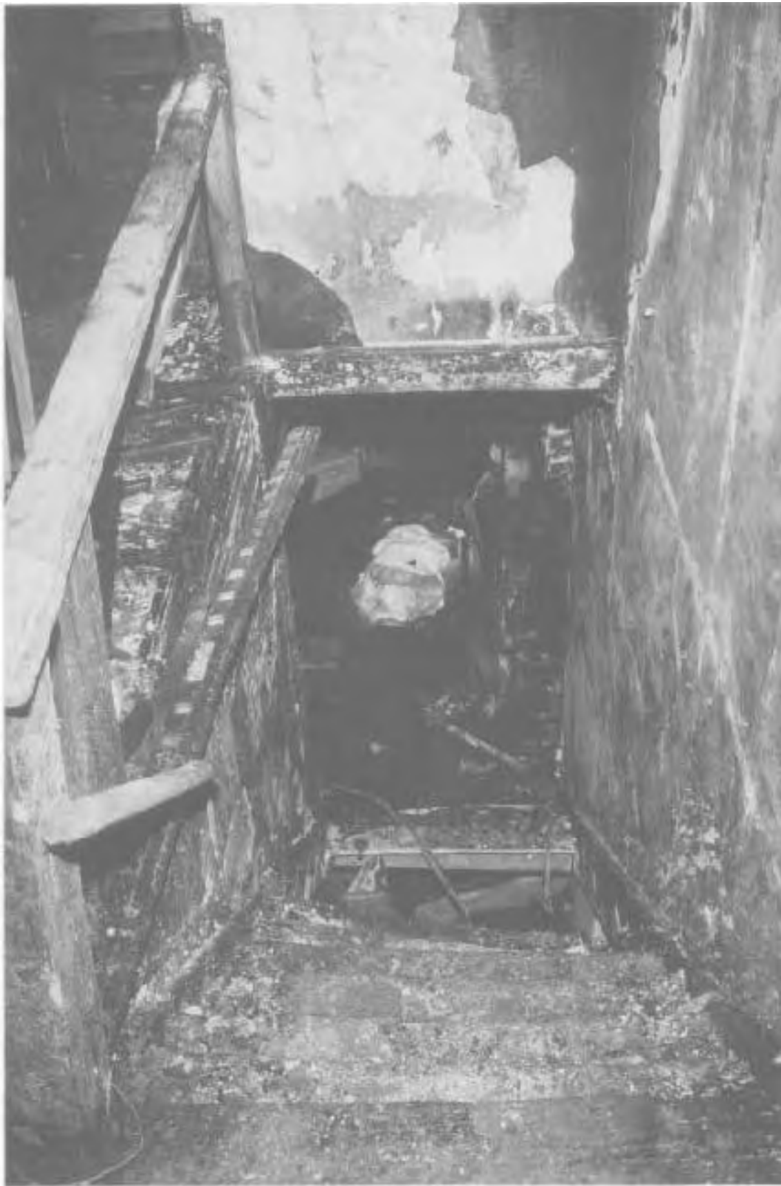
View of east side front stairway looking down from second floor. Although heat damage is slightly less intense here, evidence of extensive heat and smoke spread is clear.
