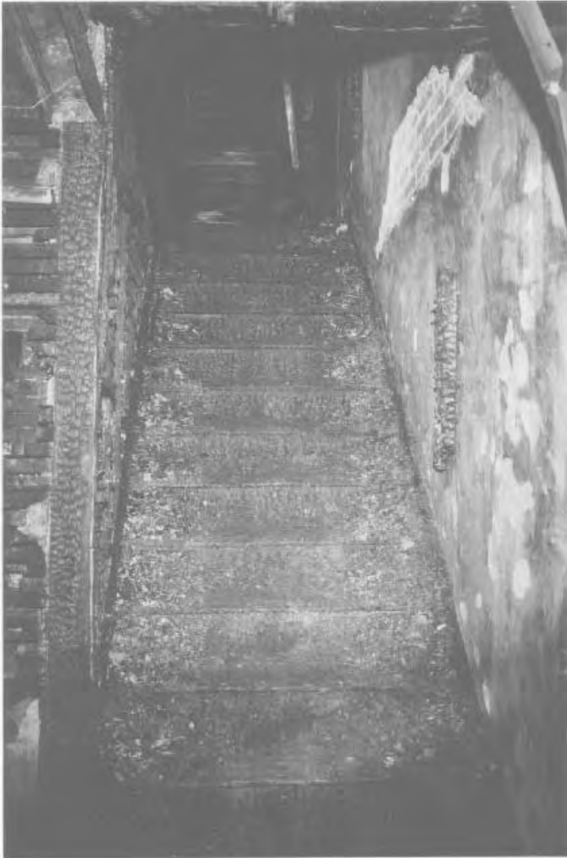
West stairway leading from the first floor living room to the second floor shows extensive charring to the stair risers, evidence of intense radiant heat exposure as the fire spread vertically cutting off the egress path.
