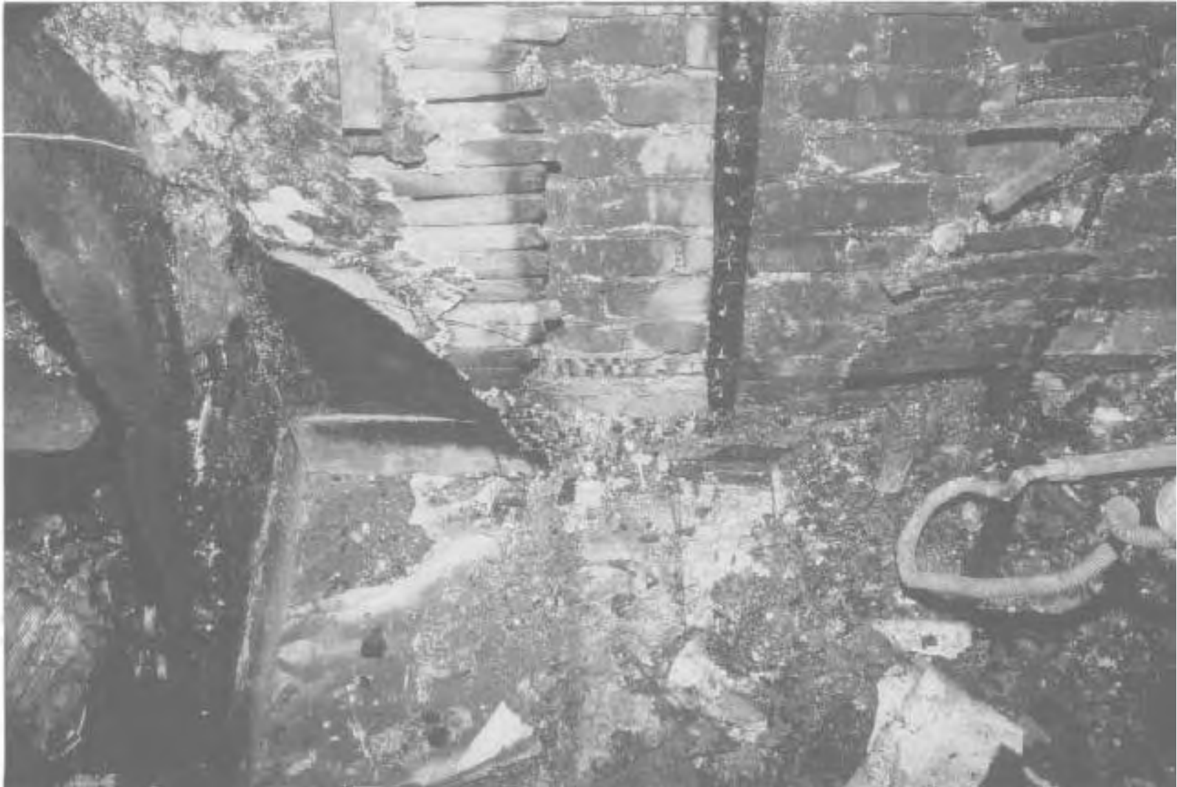
Close-up of the point of origin. A small triangular section of the particle board installed over the plaster and lath remains in the lower center portion of the picture.
