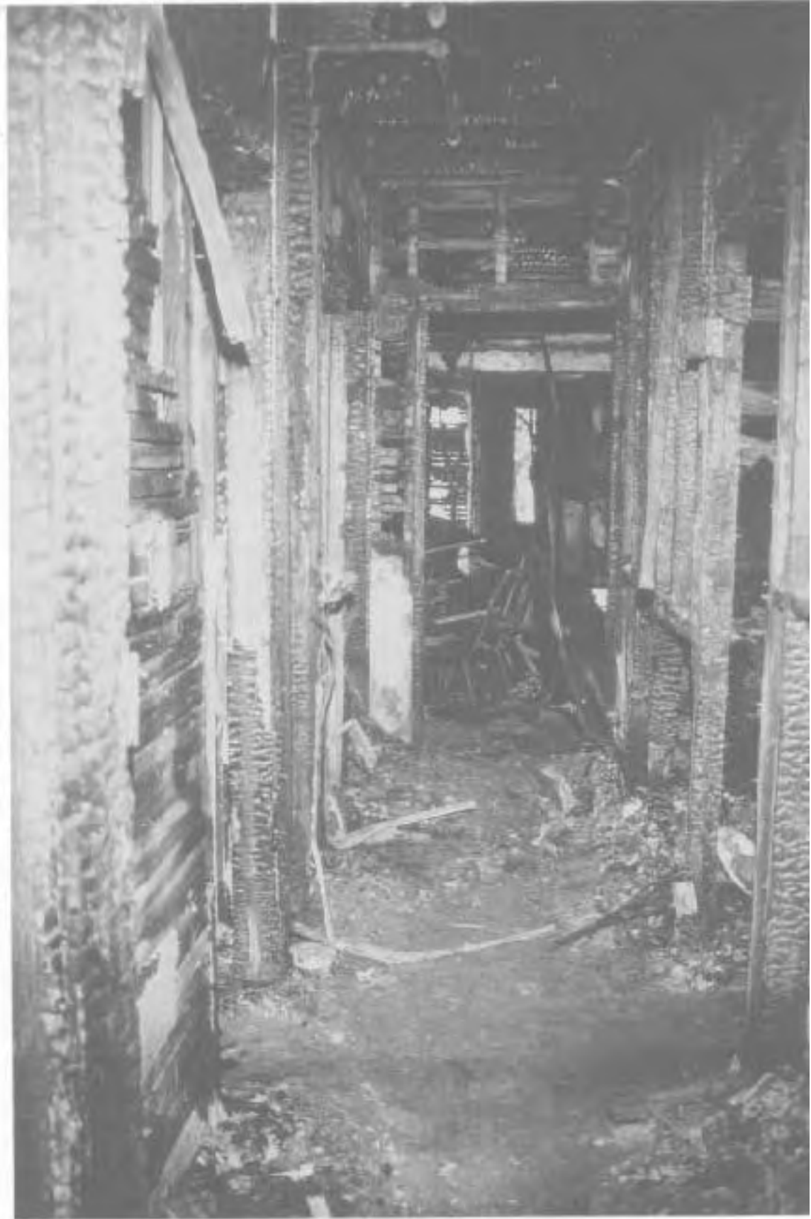
View looking south down the rear corridor adjacent to the kitchen showing heavy damage to the wall studs near the floor level. Also visible through the door opening at the south end of the corridor is heavy fire damage in the dining room.
