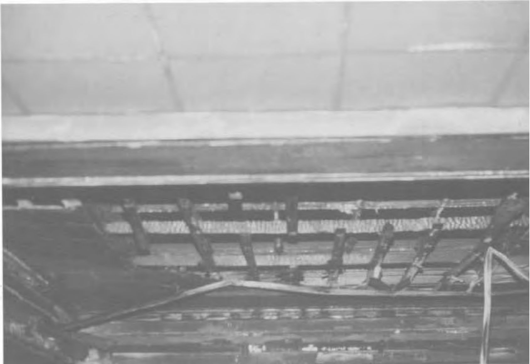
View of suspended ceiling damage above the location in the grill room where Captain Spalding was found unconscious and covered in debris.
