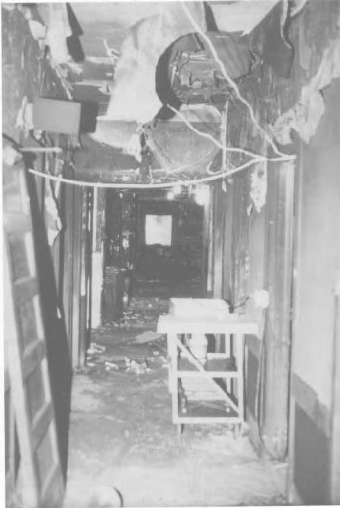
View of third floor service corridor looking east from standpipe cabinet. Note the relatively minor damage. Most of the damage is confined to wall and ceiling finish materials.
