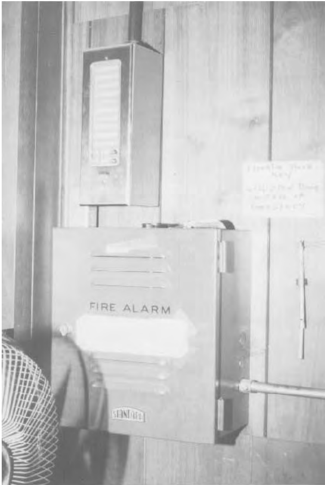
Manual fire alarm system cabinet and tabular fire alarm annunciator above. This system provided power to the fire alarm signals on all floors.
