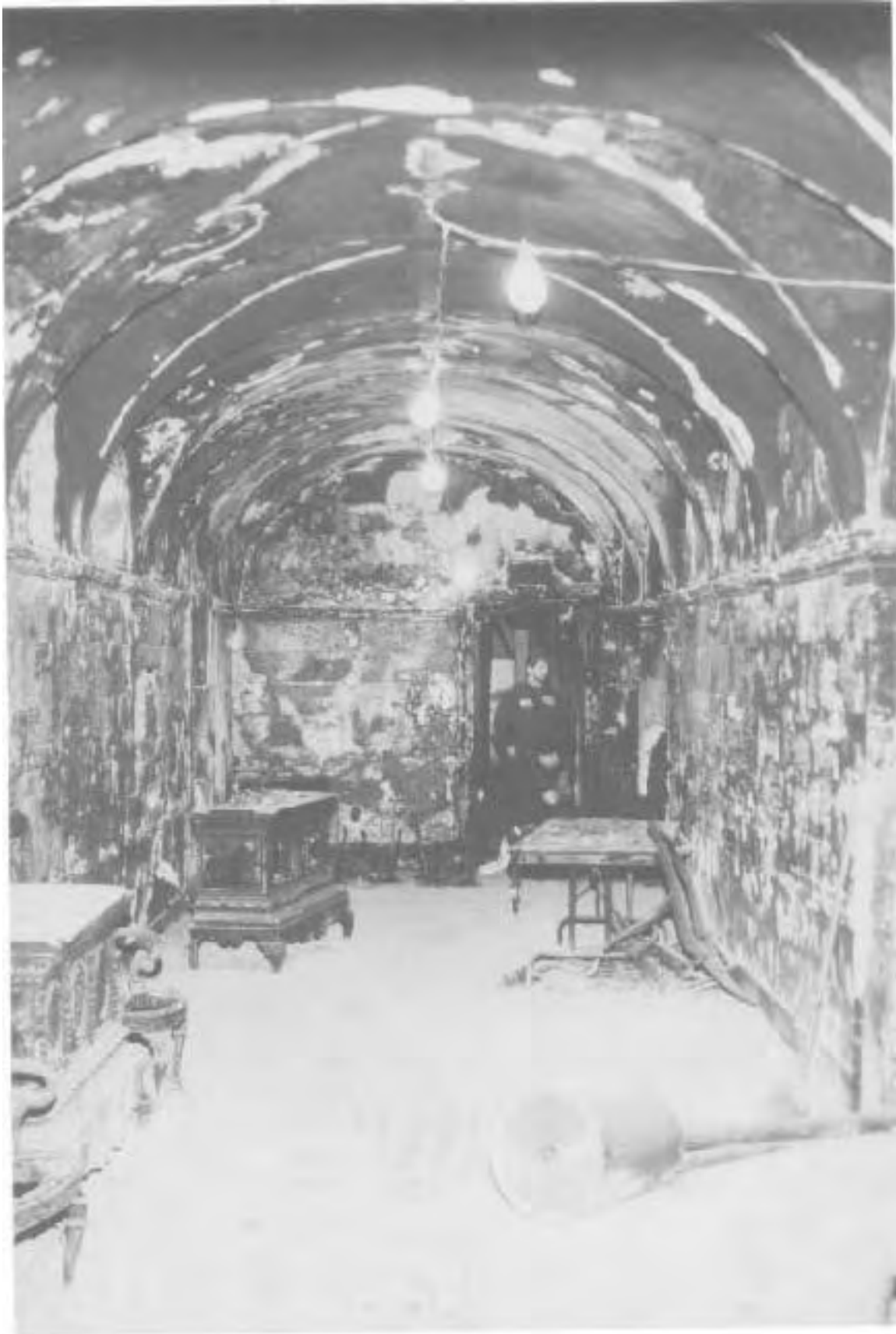
View of fire damage in the fourth floor corridor looking west toward the center of the building.
