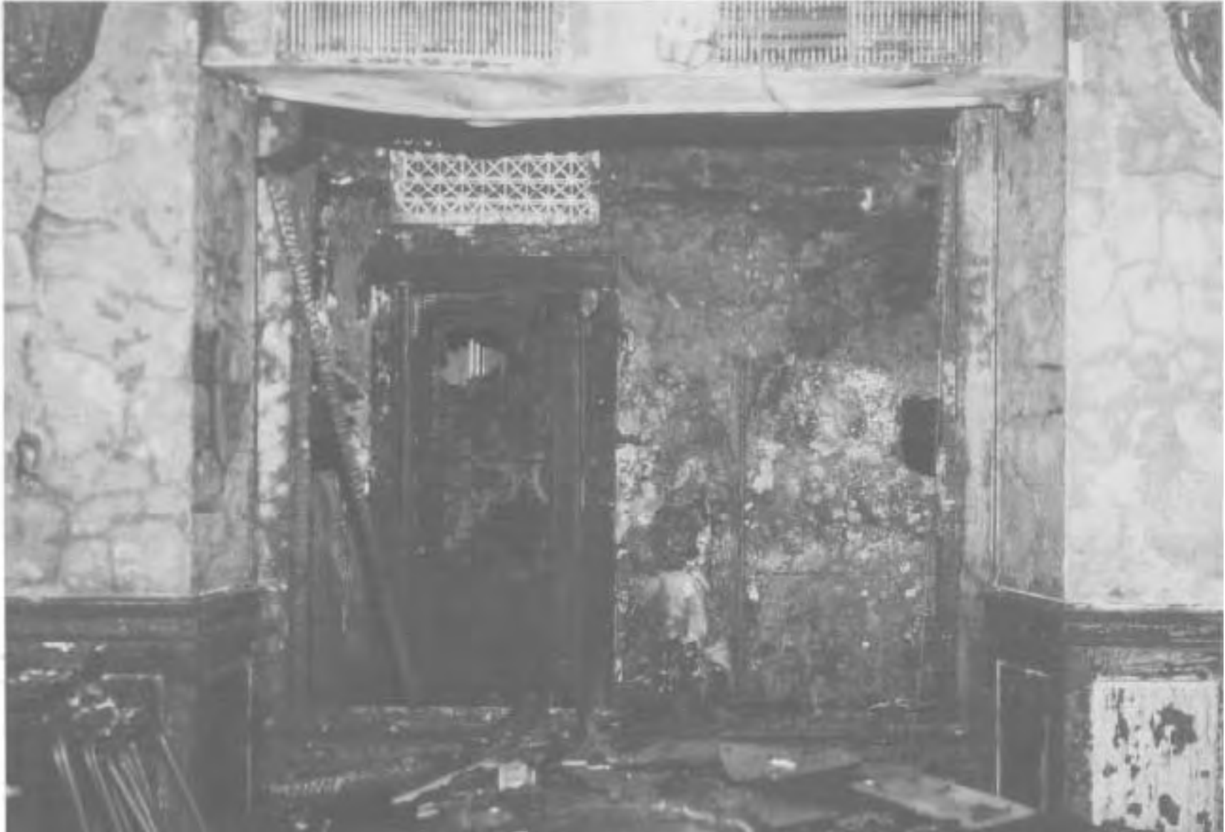
Entrance to ladies room adjacent to the dutch-style service door to the bar (room of fire origin). Note the air return register over the door and the air supply register over the opening to the dining room.
