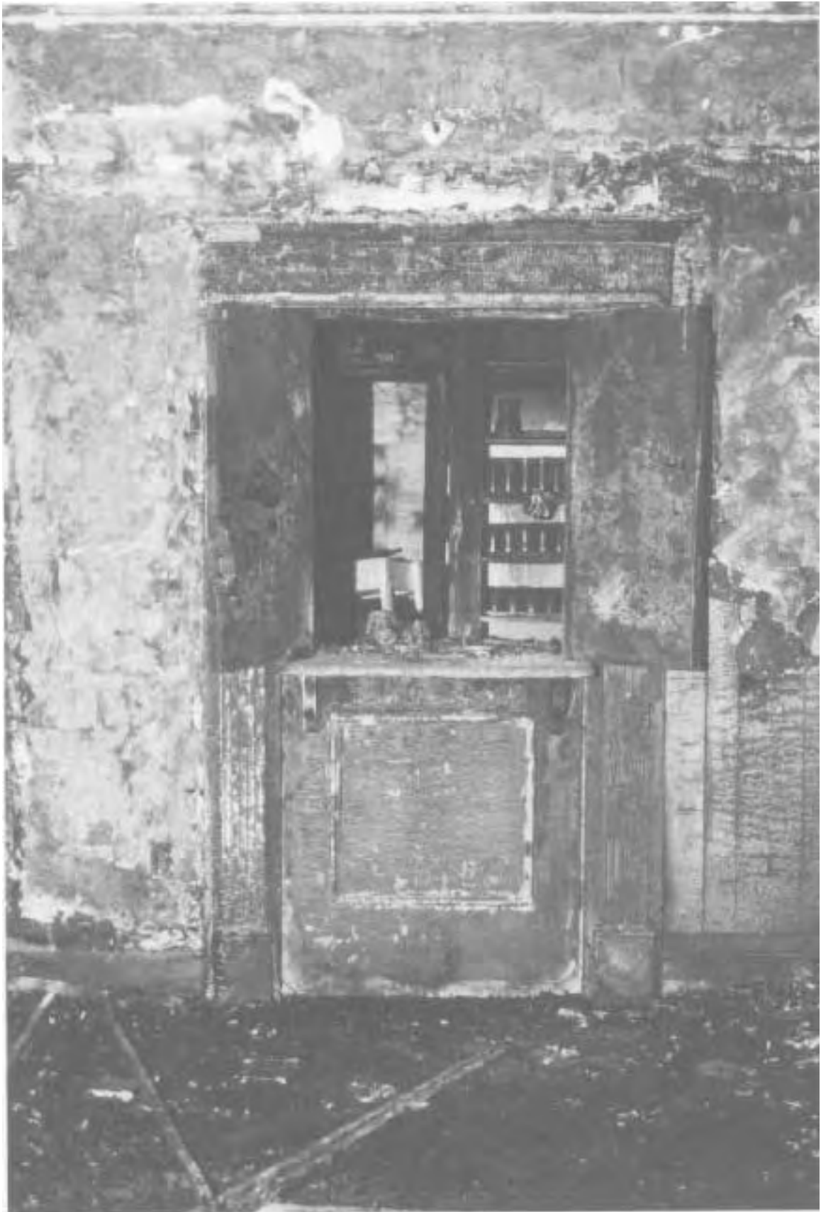
This view of the dutch-style service door to the bar room shows the deep charring to the door frame above the opening and the plywood paneling on the lower right side of the door opening.
