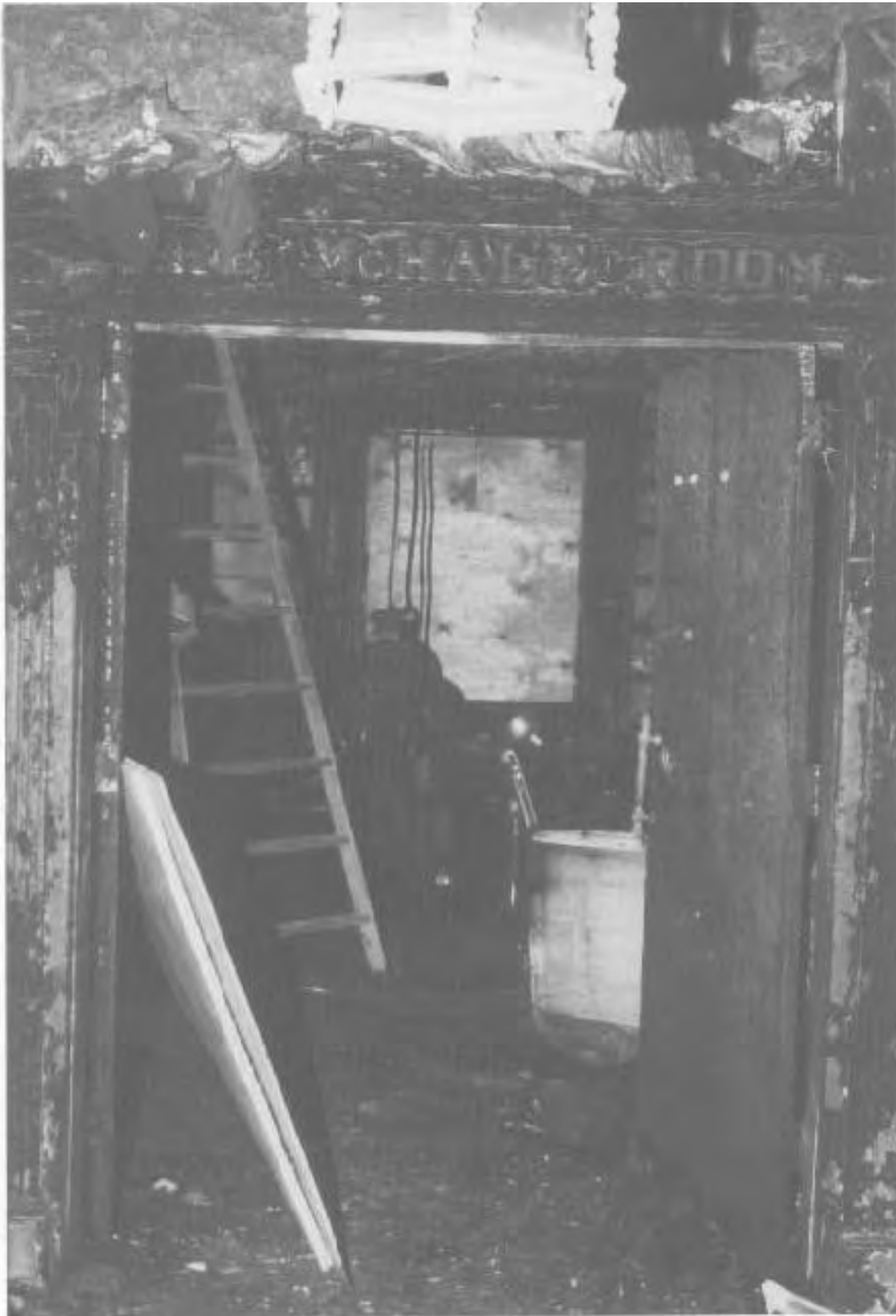
Entrance to the McHale Room looking north from the elevator lobby. Note the fire damage to the wall coverings above the door and the relatively light charring of the door frame.
