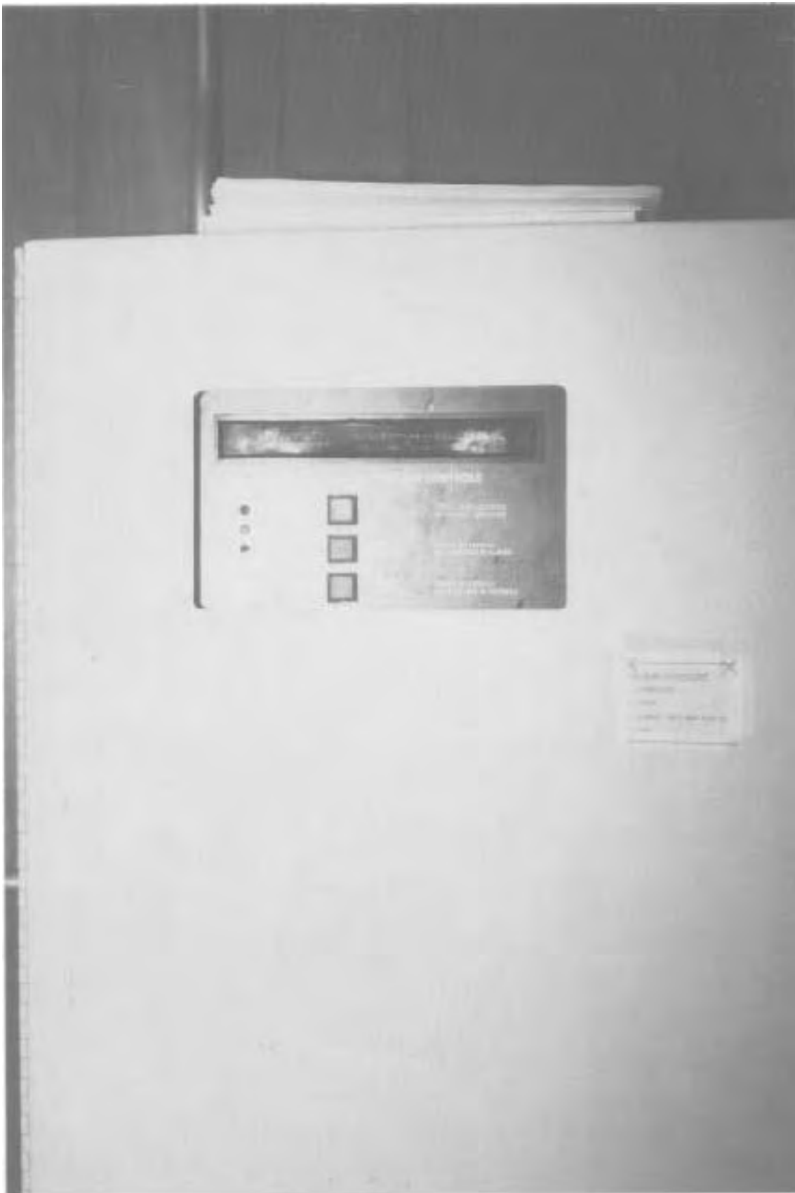
Analog addressable smoke detector control unit. This unit powered and supervised the in-room and basement smoke detectors as well as monitoring the conventional zoned control units which powered the corridor smoke detectors.
