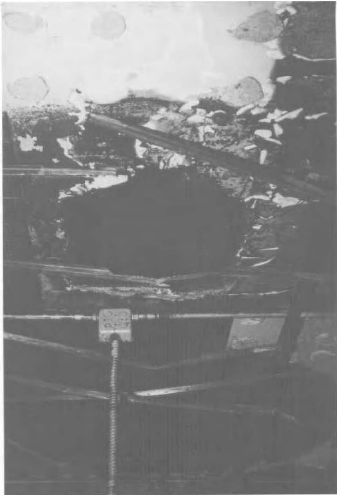
View of opening in suspended ceiling in the McHale Room. Note the charred 1-foot ceiling tiles (at left) glued to the underside of the plaster suspended ceiling and the remnants of the aluminum suspended ceiling frame.
