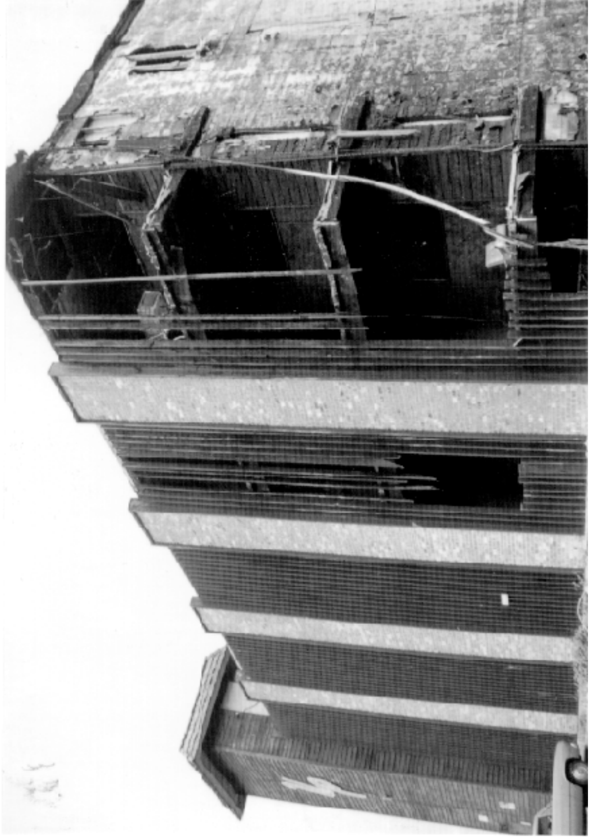
(Photo provided by Philip Schaenman) Close-up of west facade of Building A; its southwest corner was damaged.
