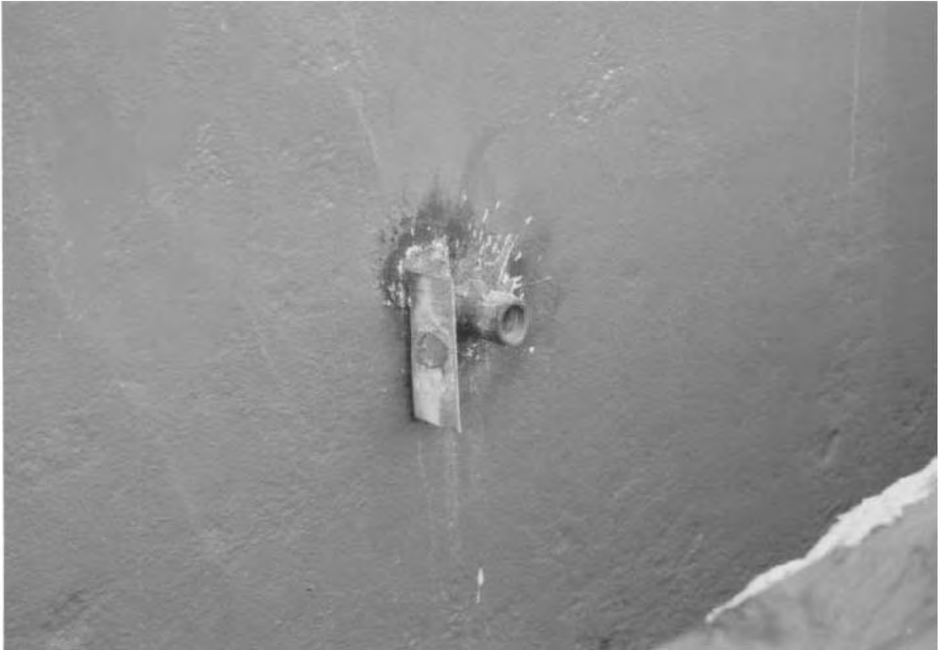
Closeup of hole used to insert CO 2 , with coupling welded into place.
