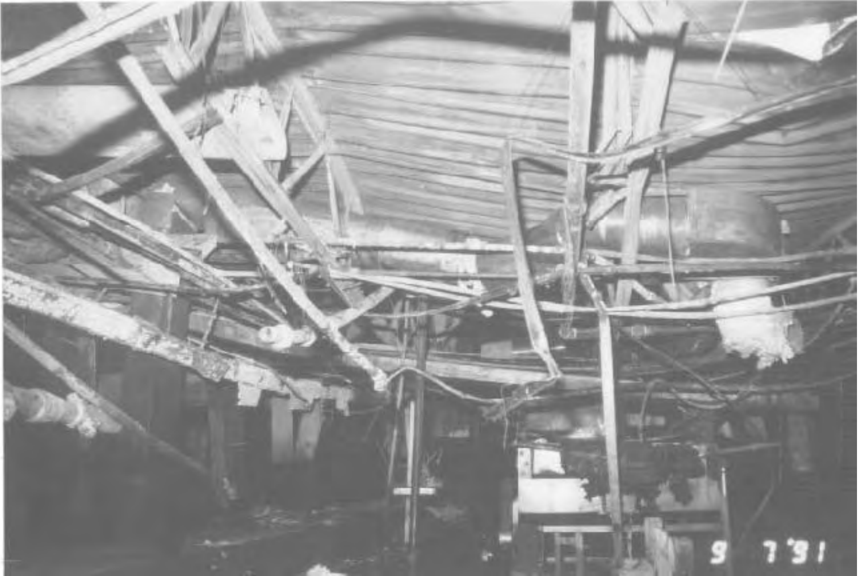
Damage to the steel girders and roof supports over the area of origin.
