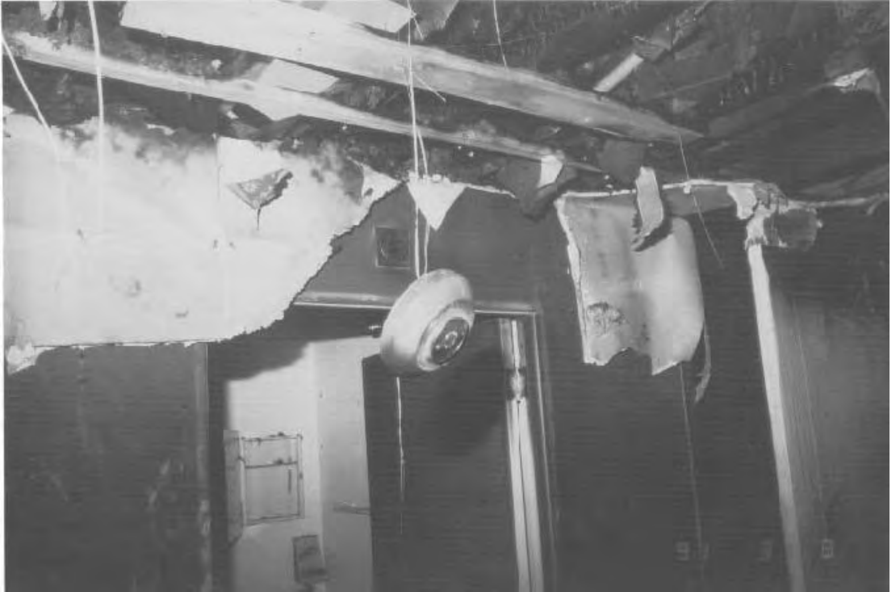
Older existing smoke alarm in the structure, hard-wired, no battery backup.
