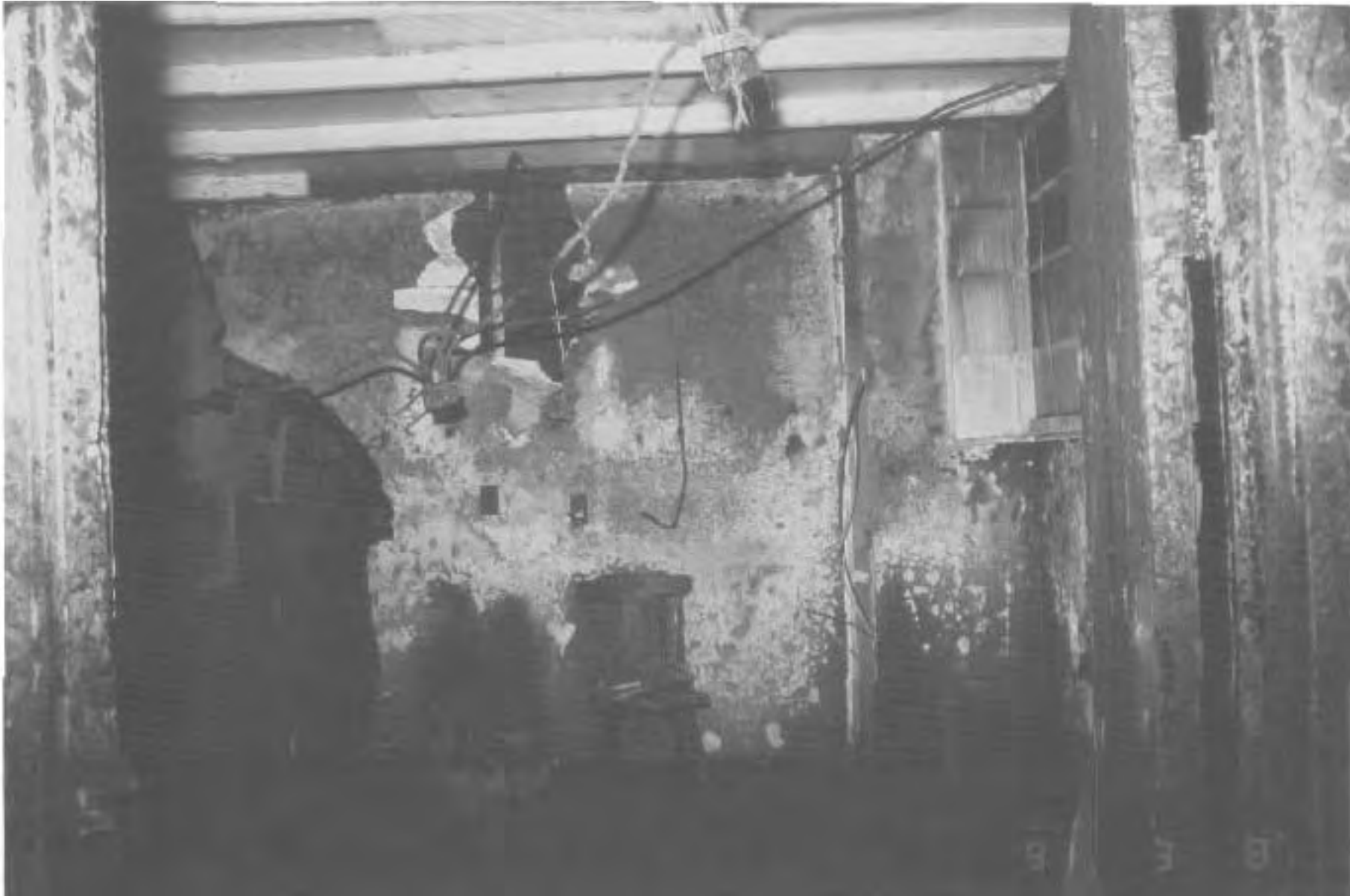
The smoking room. The corner to the right is the northwest corner where the vent stack to the heating unit below is located. This was thought originally to be the Area of Origin.
