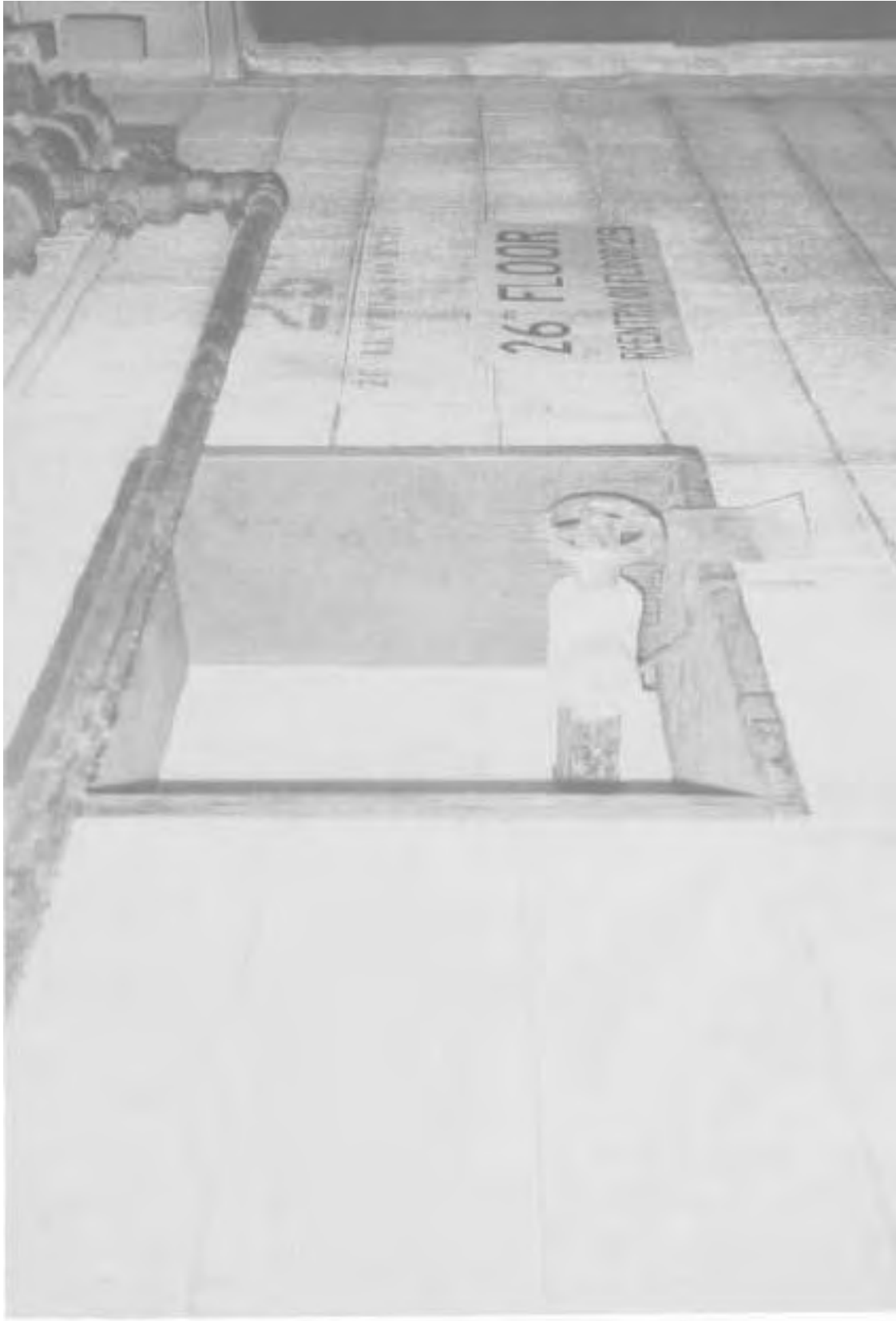
Standpipe hose outlet with pressure reducing valve (PRV), 26th floor.
