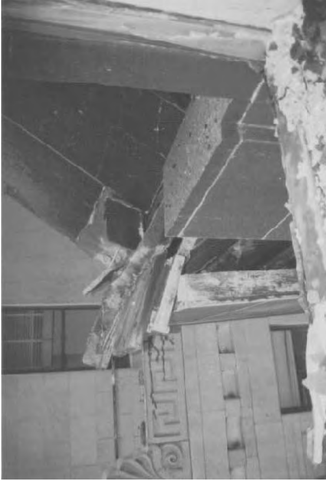
Here and in the next two photos exterior granite panels from the east stair tower were dislodged due to the thermal expansion of the steel frame of the building.
