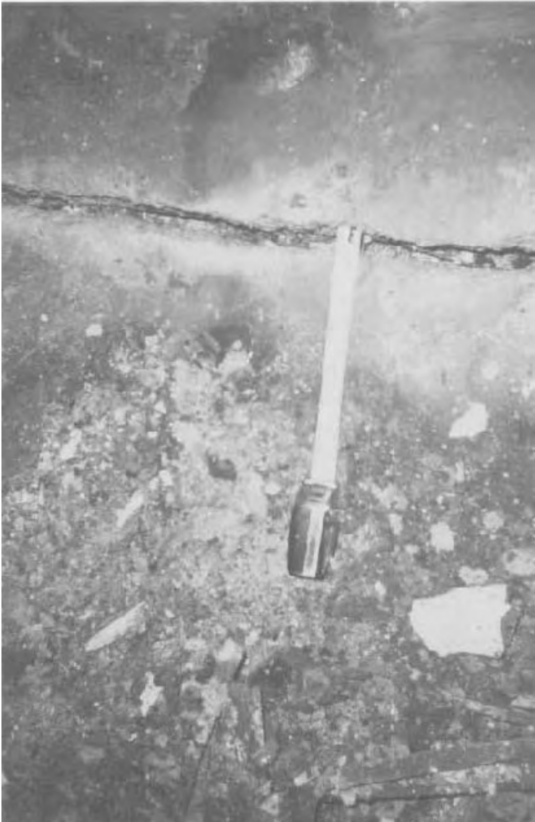
Close-up of crack in concrete floor, 28th floor.
