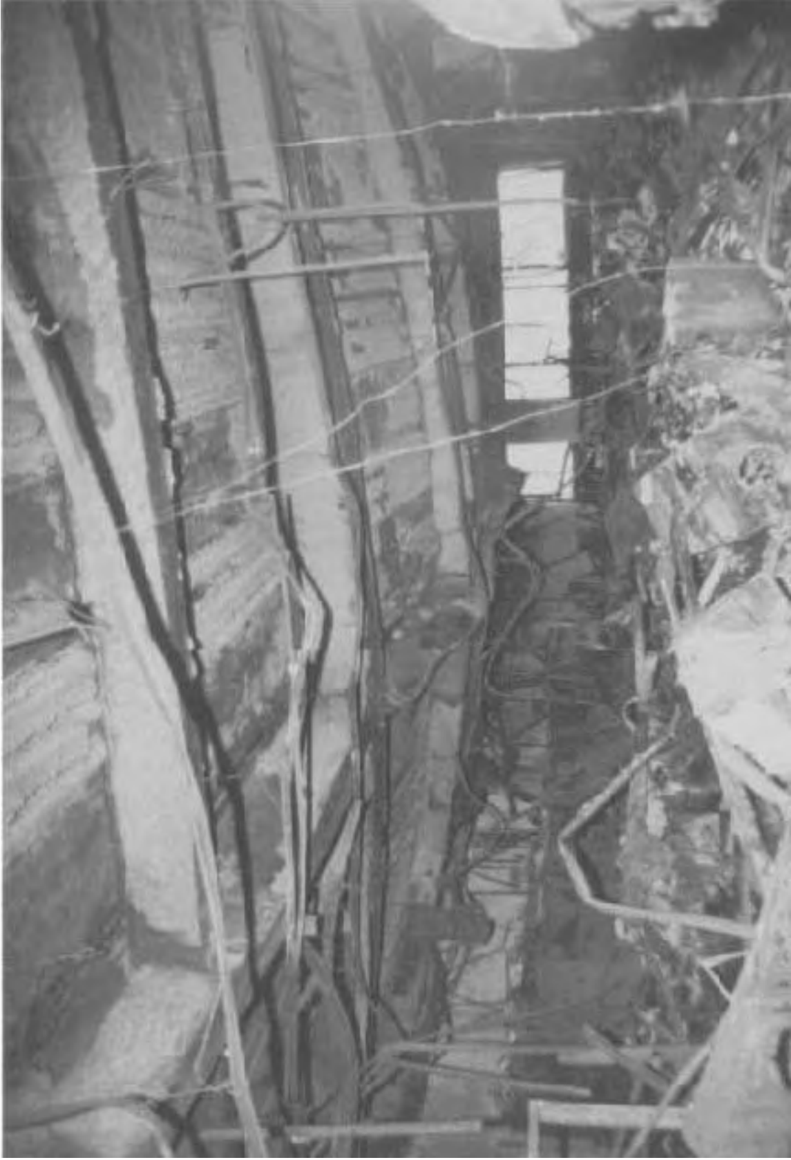
Here and in the next three photos are interior views of floor areas after the fire. Note the total consumption of the available fuel and sagging of the floor deck of up to three feet between columns.
