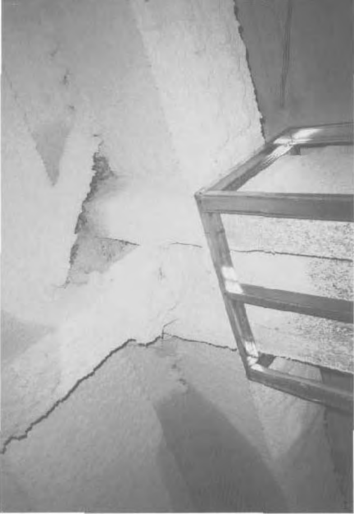
Detail of typical Type 1B construction, 6th floor. Note the spray-applied fireproofing and framing for gypsum wallboard.
