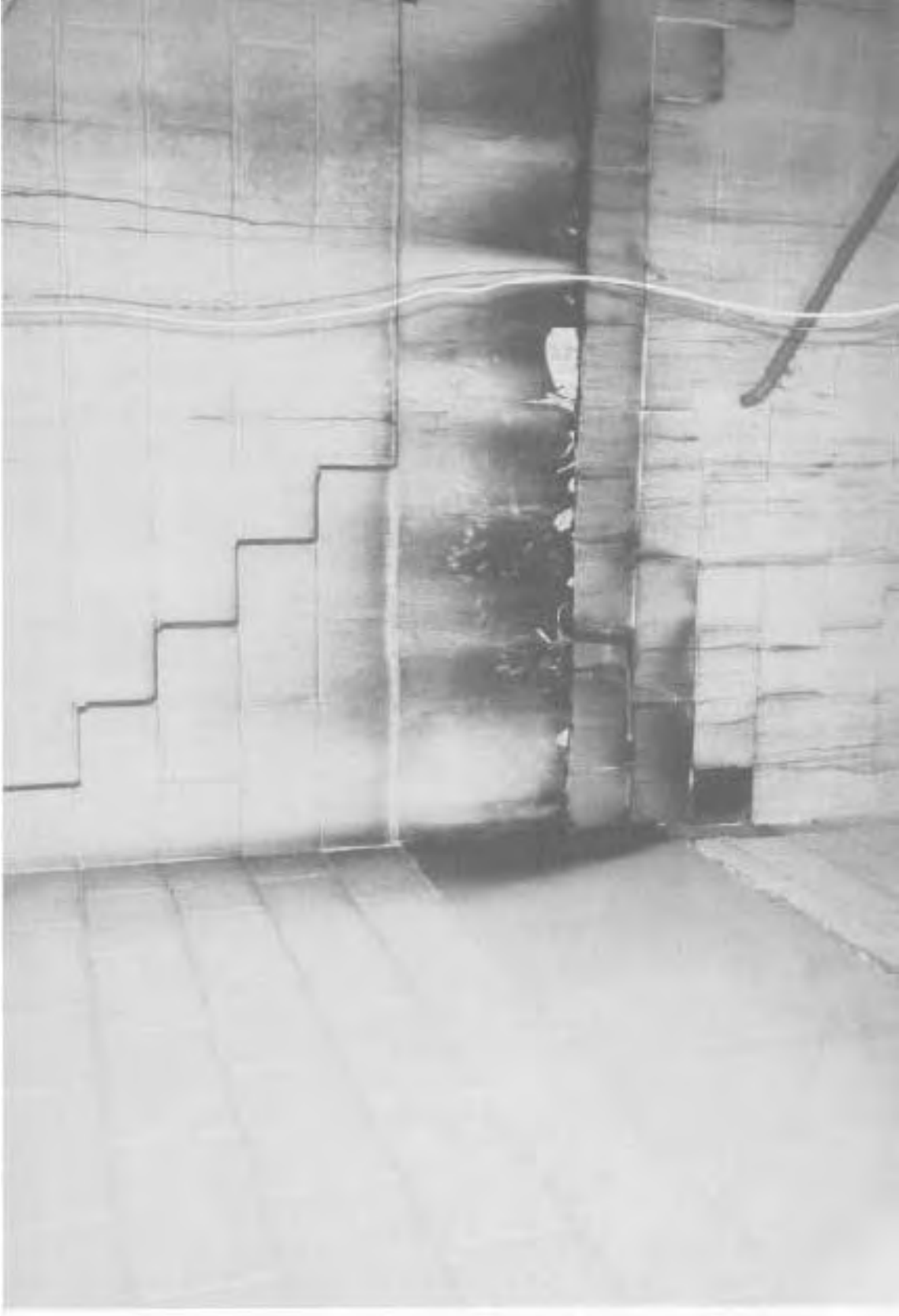
Fire tower between 25th and 26th floors. Note heavy fire and smoke damage.
