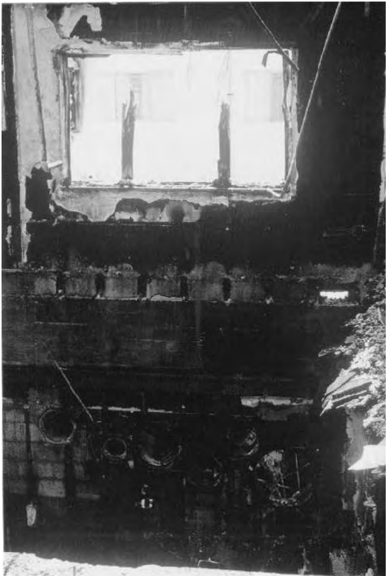
Second floor, looking across to Room 301 from front stairway, area of origin is at base of photo.
