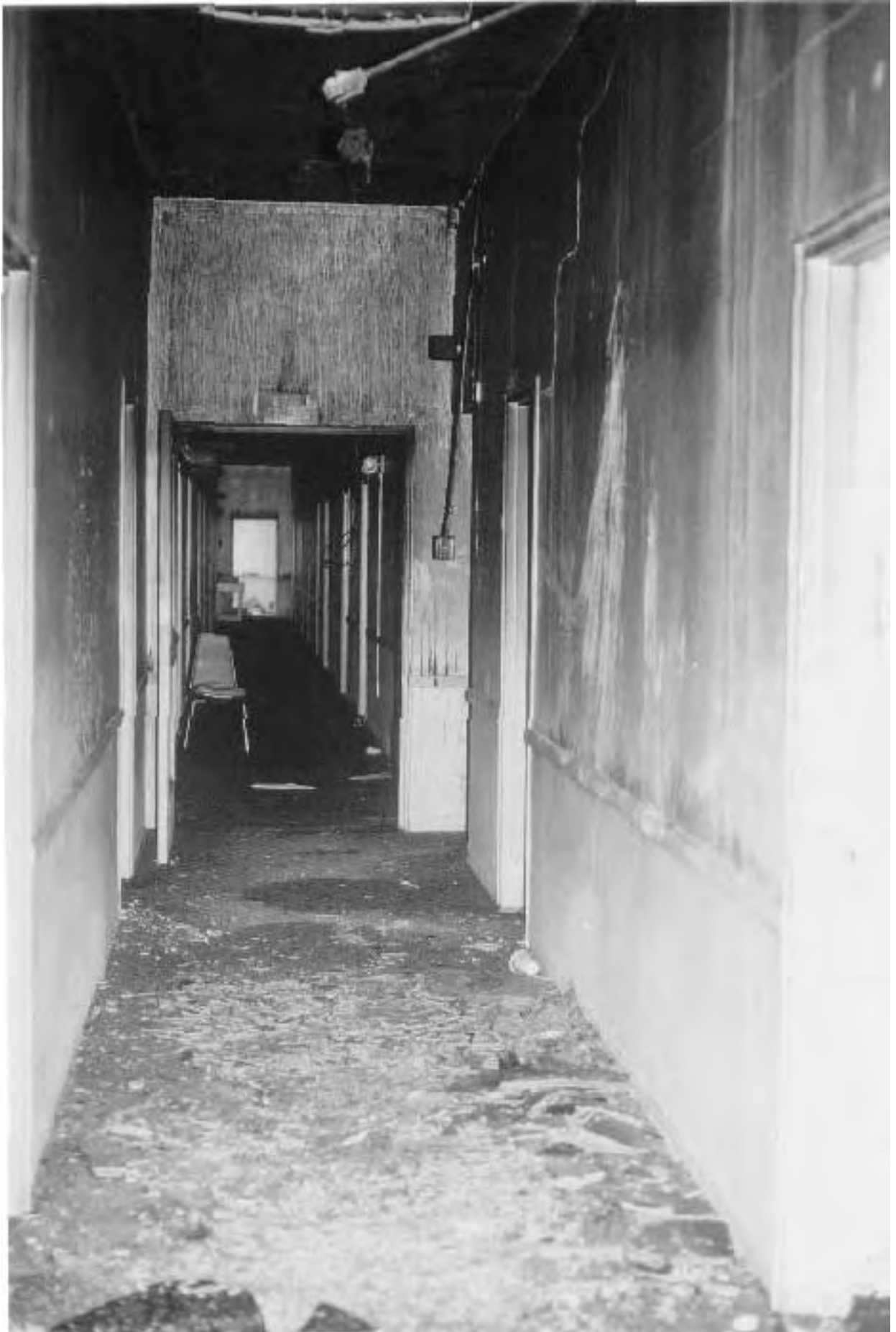
First floor corridor, looking to rear of building from lobby. Fire door in foreground was closed throughout much of the fire.
