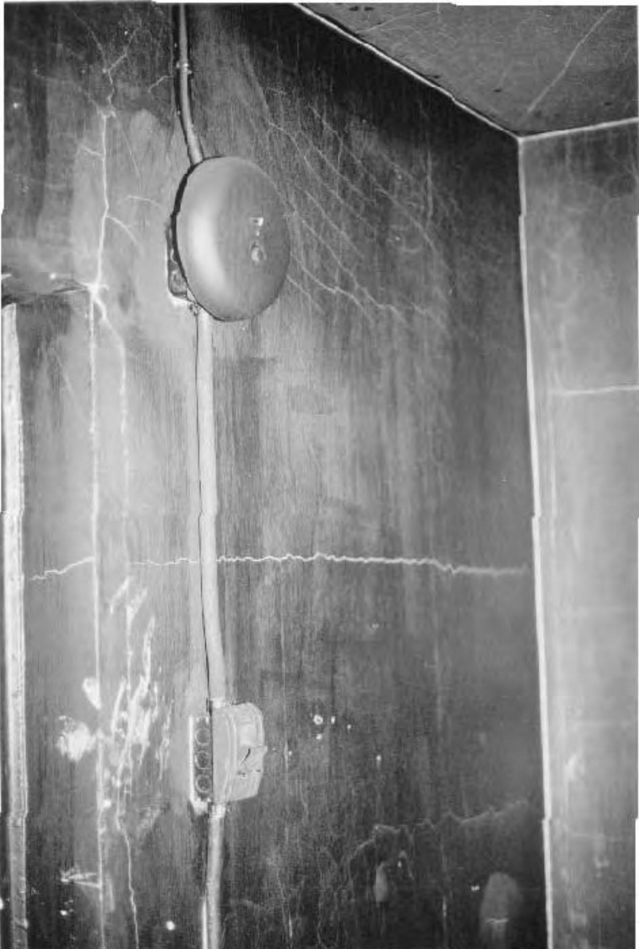
Manual fire alarm station and bell, third floor, at rear stair. Note extensive darkening soot.
