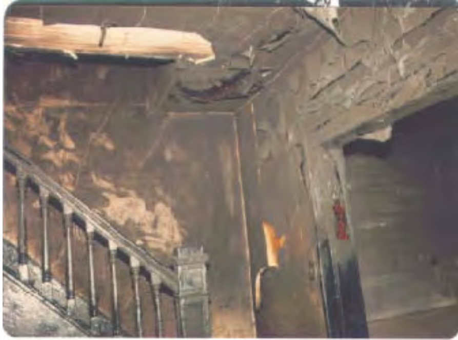
General location of the smoke detector at the base of the stairwell.
