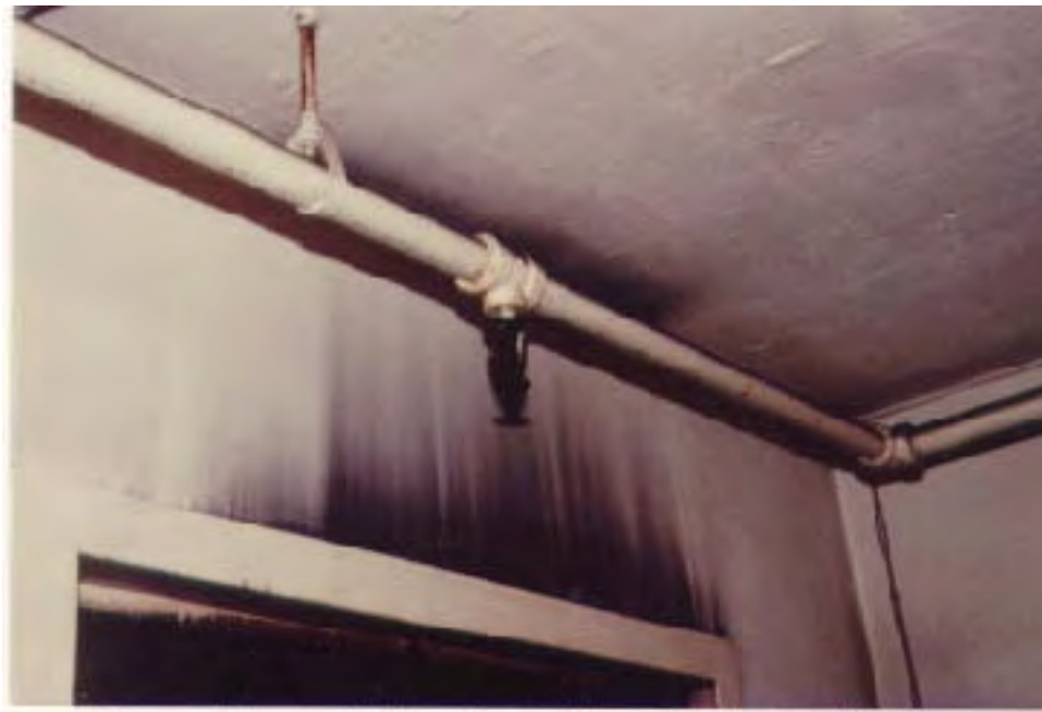
Figure 15. Sprinkler in maid's closet immediately adjacent to area of origin was not activated due to performance of fire door.
