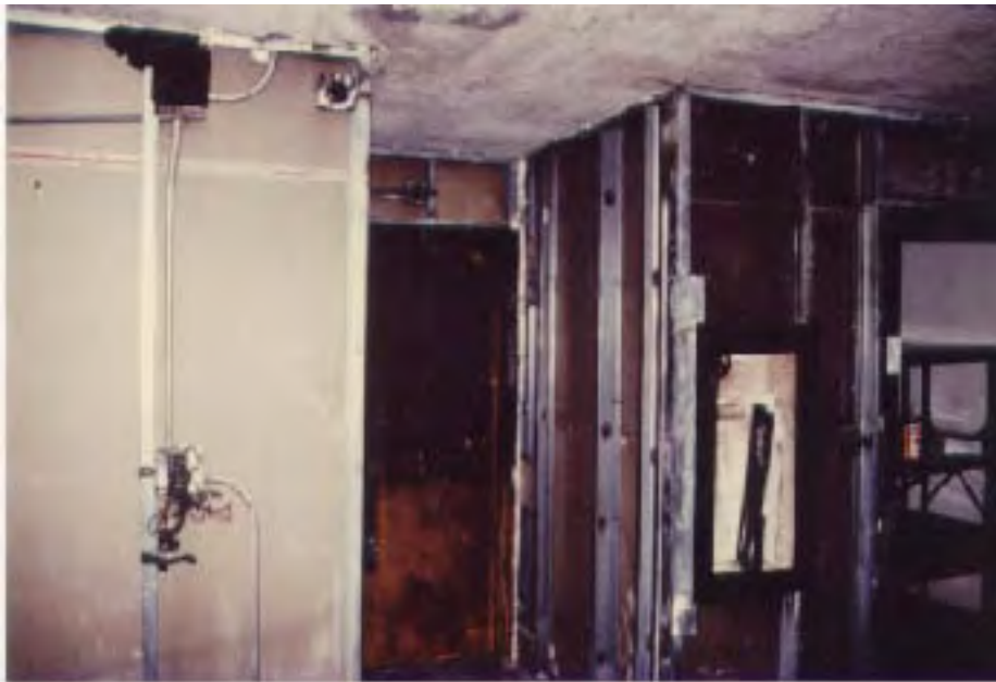
Figure 7. Entrance to exit Stairway 2 -- 10th floor. Note pull station at left used to initiate local alarm by guard.
