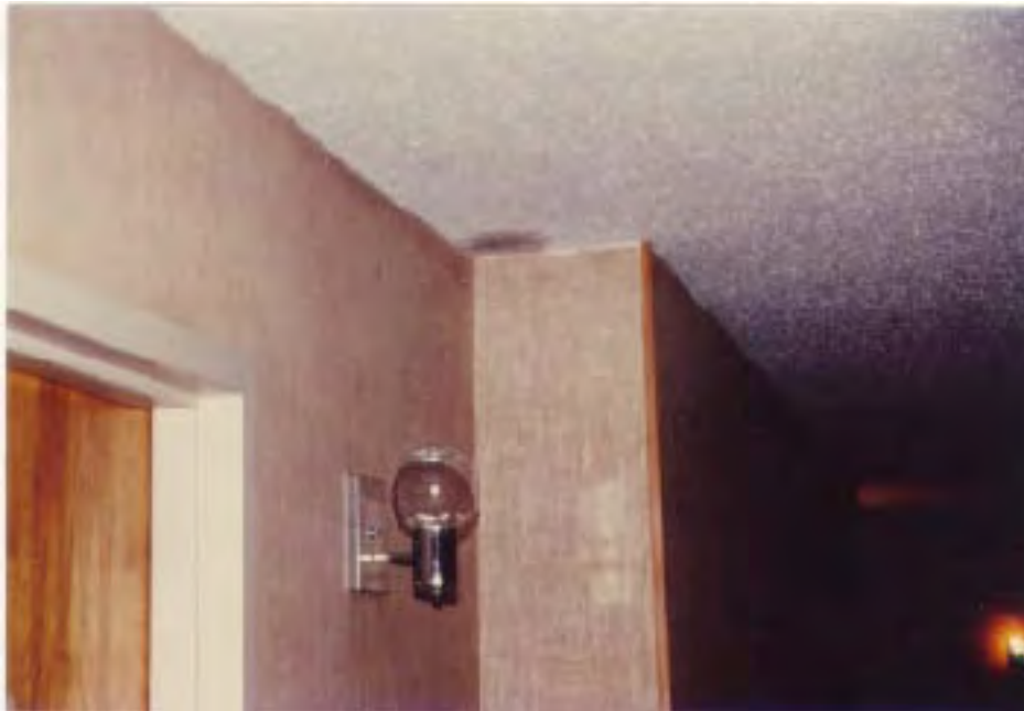
Figure 12. Location of corridor smoke detector (dark spot on ceiling).
