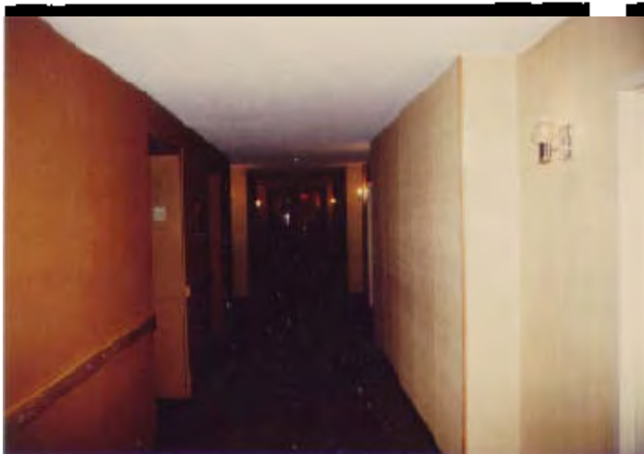
Figure 5. Entrance to exit Stairway 1 -- 10th floor. Note the ventilator opening (upper left) and fire hose/extinguisher cabinet (lower left).
