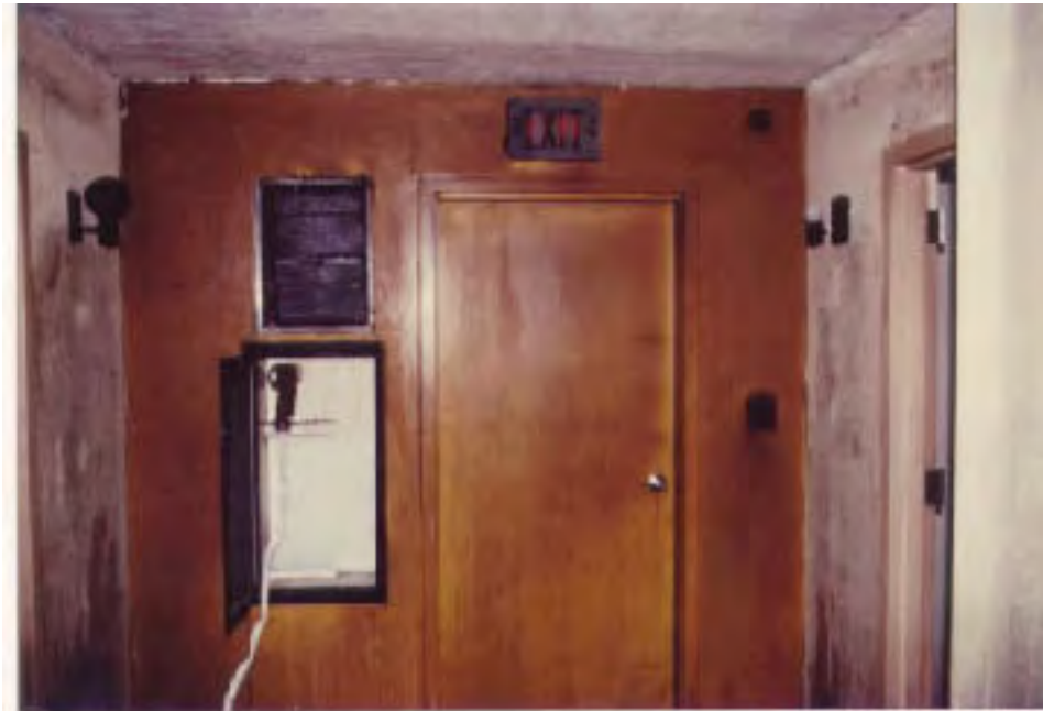
Figure 4. View of short corridor from area of origin toward Stairway 1 -- 9th floor.
