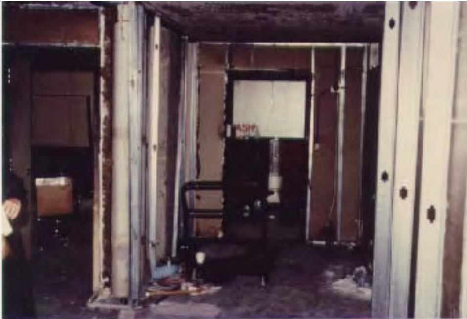
Figure 9. Area of origin on 10th floor.
