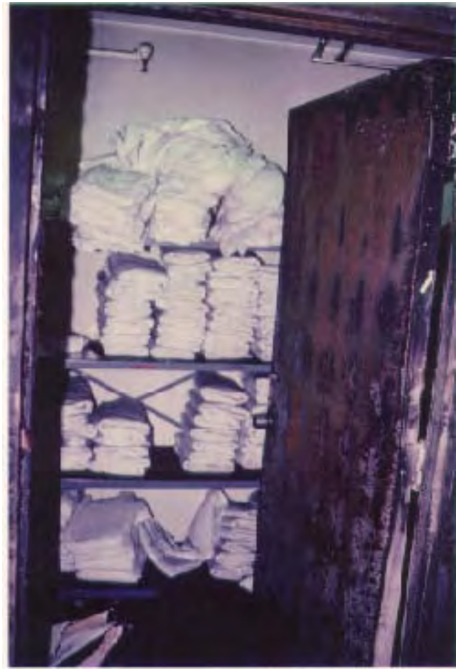
Figure 14. Fire door protected linens in closet only 20 feet from area of origin.
