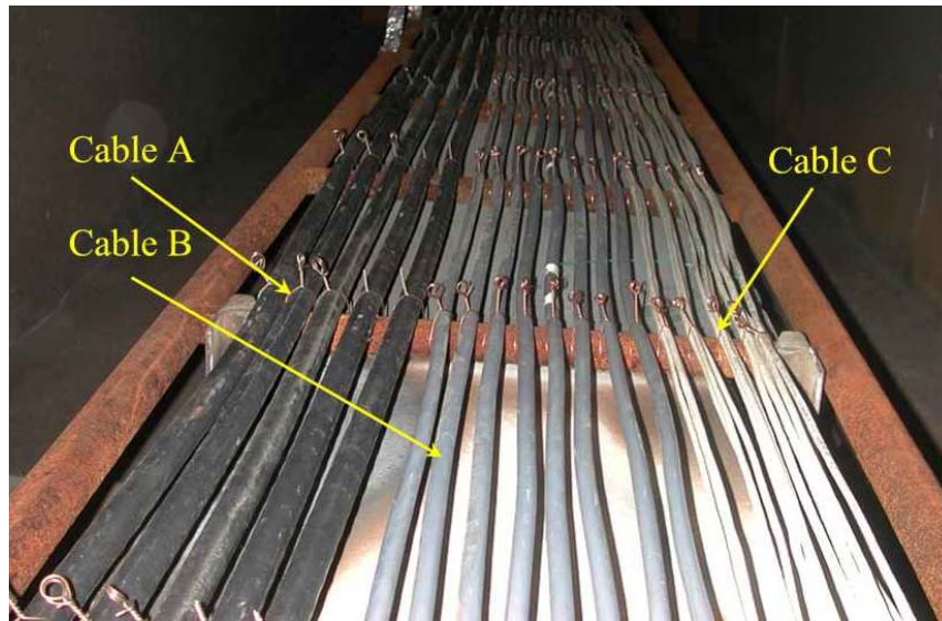
Figure 15. Mounting configuration in the vertical tests, first series. The white backing board is visible behind the cable ladder.
