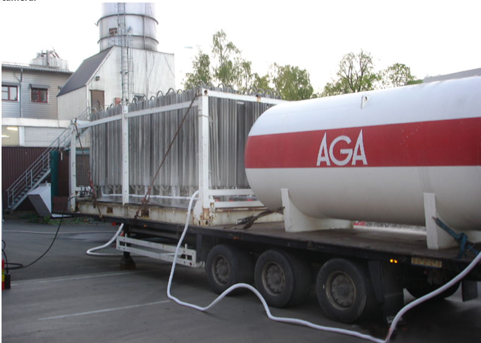
The nitrogen tank and evaporator parked by the silo.
