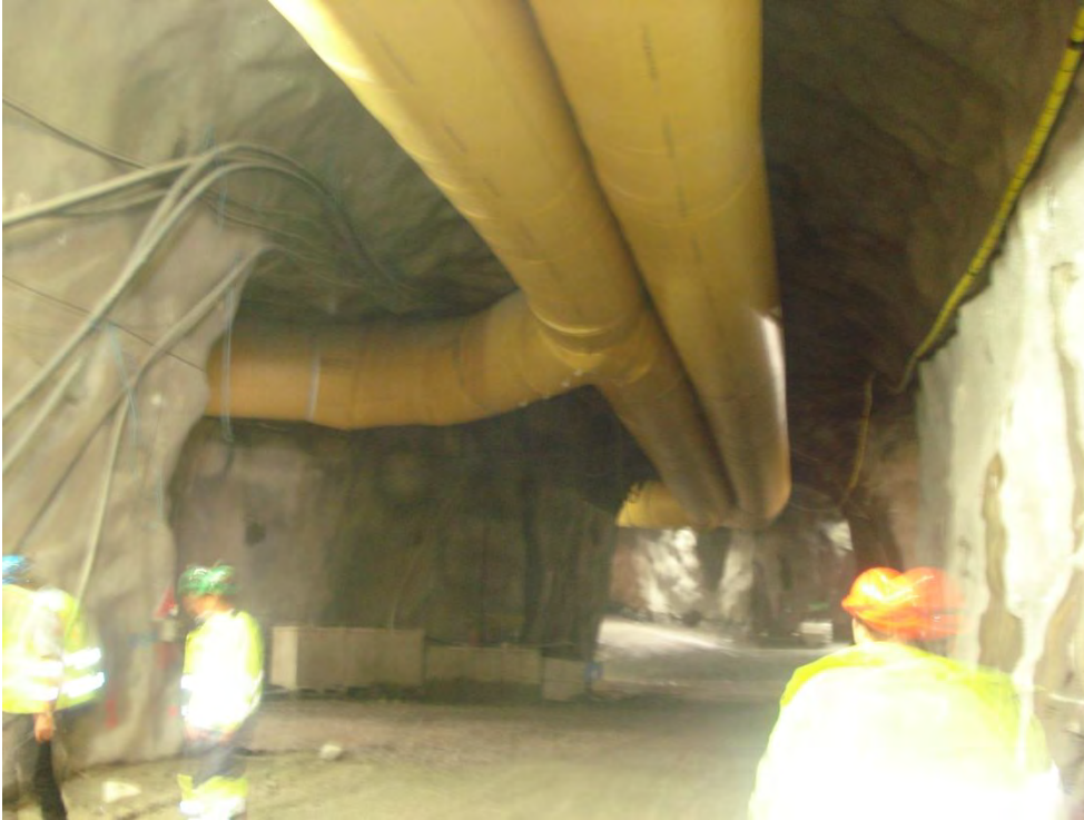
Figure A 2 The fresh air ventilation ducts in Norra Länken.
